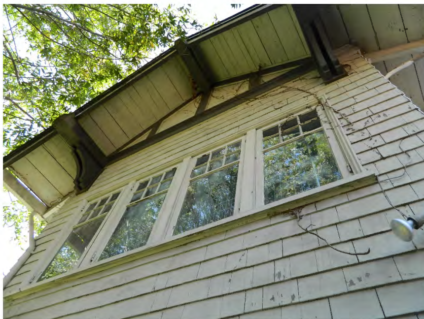
Photo showing the north elevation "ground floor" gable with knee braces and gable timber detail.
