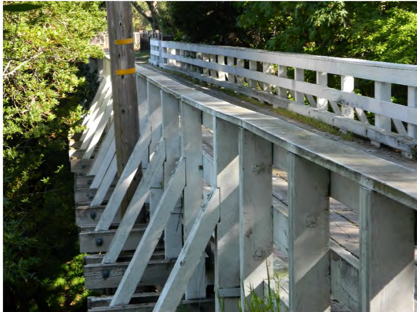
Photo showing the east side at the north approach to the bridge, facing south.
