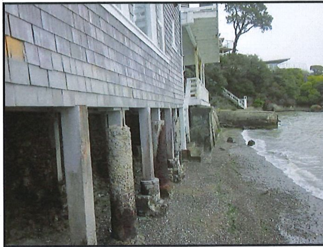
Figure 2: The Beach Drive/Oak Drive beach sewer is under water at the right side of the picture.
