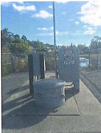
BEACH FIBERGLASS PUMP STATION
