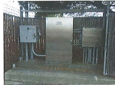
THIRD STREET PUMP STATION
