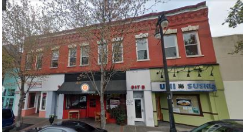
813-819 4 th Street (APN 011-273-04). Mapped as a contributor—rated B. Apparently built in 1908 and is in good condition.
