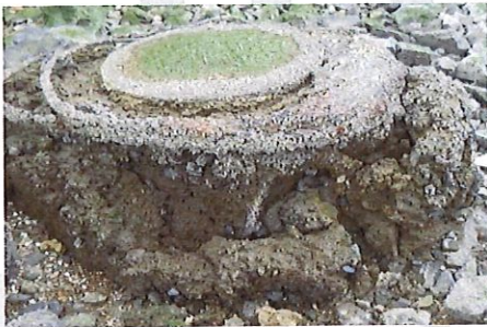
A corroded manhole in the Bay.
