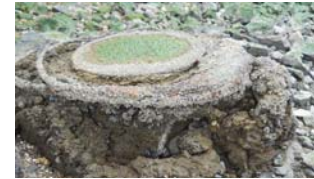
A corroded manhole in the Bay.
