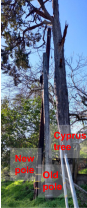
Figure 4. Soil subsidence and creep. The picture is taken where Ross Street Terrace, lot 45 (62 Woods Street), and the proposed driveway of lot #59 intersect. Note that the old utility pole and the cyprus tree are leaning in parallel to one another, while the new utility pole stands upright. Tree trunks of nearby oak trees are leaning in the same direction as the pole and the cyprus, demonstrating soil subsidence and creep. While only one location is shown here, indications of subsidence and creep can be seen in multiple locations on and surrounding the project site.
