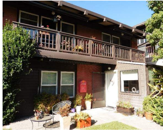
Figure 33. Two-story portion of south façade (right side) and sunroom addition, looking northeast.
