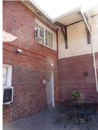
Figure 59. Close-up view of the west façade, far right bay shown with infilled brick.
