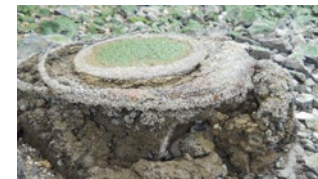
A corroded manhole in the Bay.
