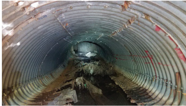
Upstream view of the arch CMP culvert showing the corroded floor and bowed flow line.
