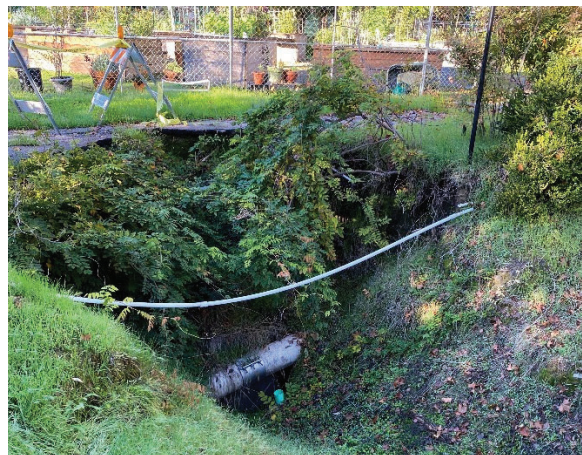
View of hole in the southeast yard of Rotary Manor. The 12-inch diameter drain pipe is visible in the hole.
