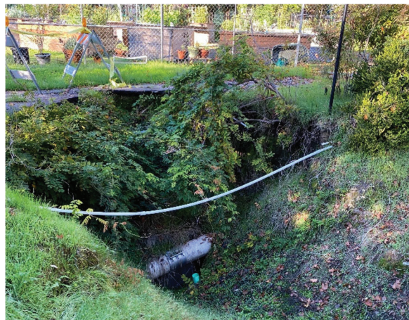
View of hole in the southeast yard of Rotary Manor. The 12-inch diameter drain pipe is visible in the hole.
