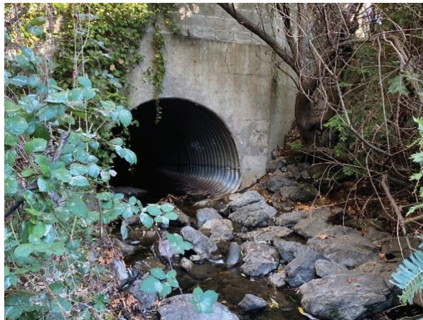
View of the endwall and open channel downstream of the CMP culvert.
