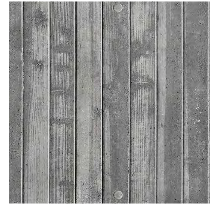
⑥ RETAINING WALLS, VERTICAL BOARD FORM TEXTURE COLOR: "GRAY W/ LAMP BLACK"
