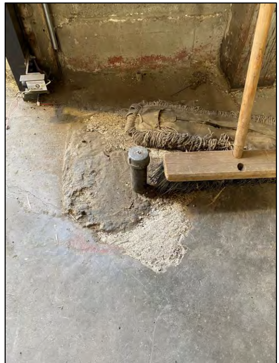
Photograph 12: Possible former fill pipe located near former waste oil UST.
