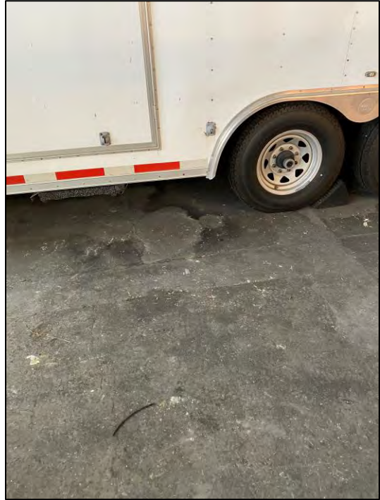
Photograph 18: Small area of staining on the concrete floor inside police storage area, likely attributable to standing water.
