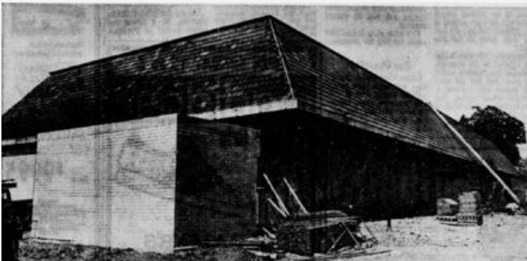
Photograph 30. Photograph of the Sears Automotive Service Center building under construction at the southern end of the Northgate Mall, 1972 (Daily Independent Journal 1972: 3)
