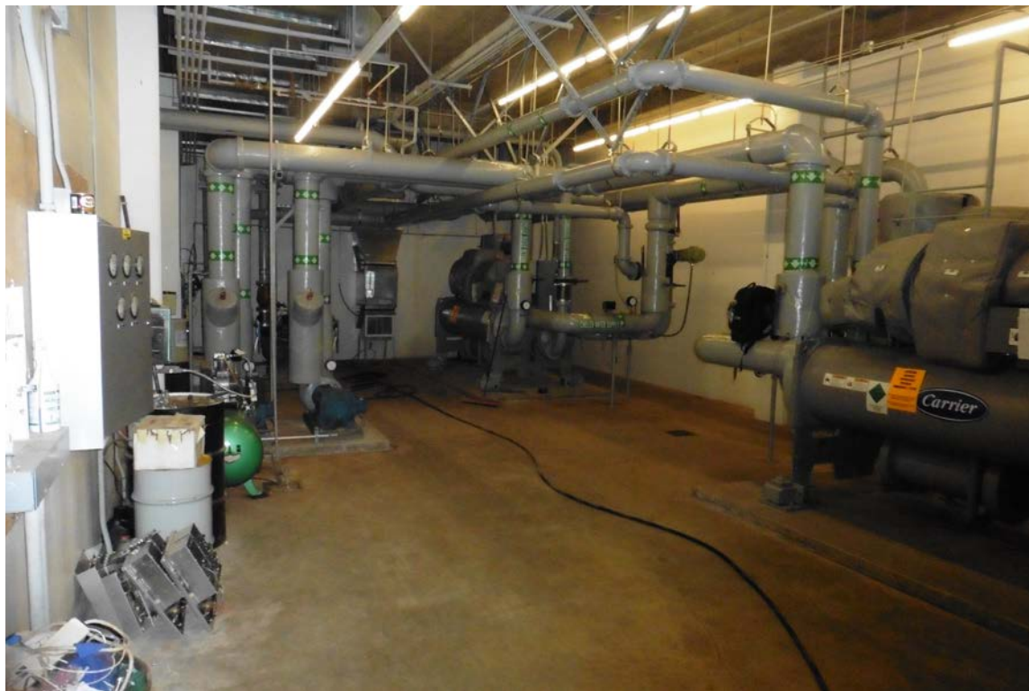
Photo 12: Chiller room, Sear's basement.
