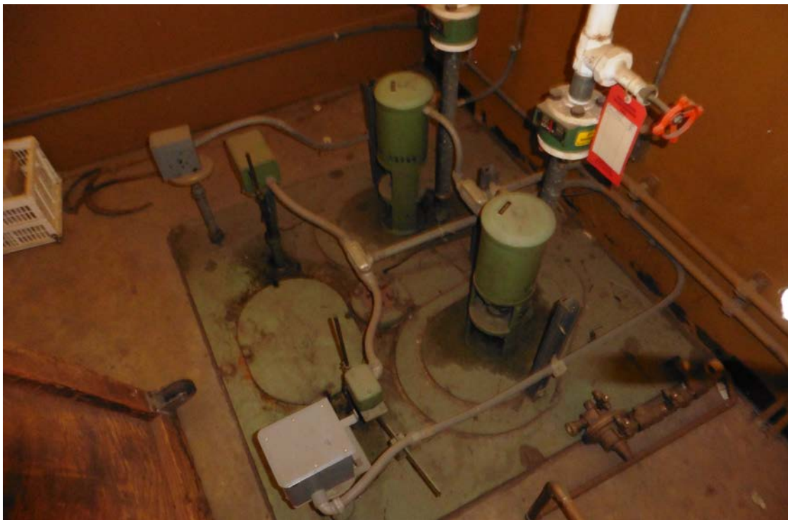
Photo 17: Groundwater pumping system in Sear's basement.
