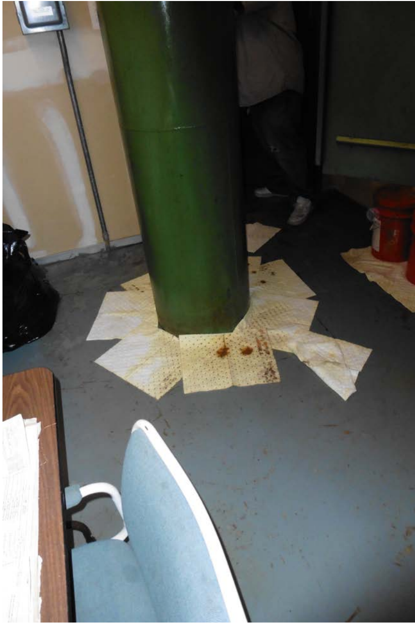
Photo 19: elevator piston casing. Note leaking hydraulic oil.
