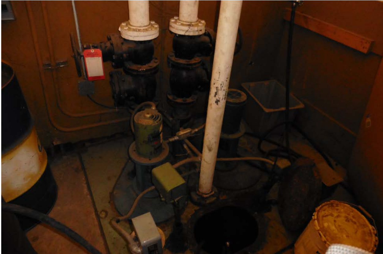
Photo 16: Groundwater pumping system in Sears basement.:
