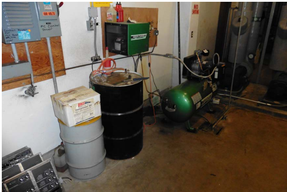
Photo 13: Air compressor and oil drum storage on concrete floor in Sear's basement.
