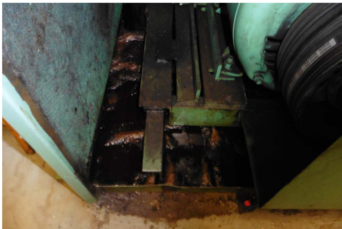
Photo 14: Hydraulic oil at elevator motor room Sear's department store basement.
