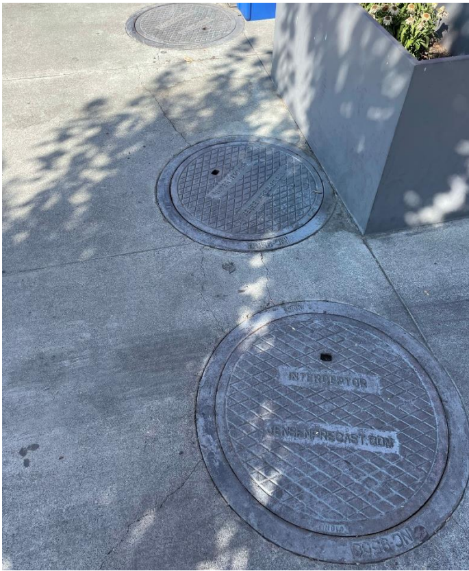
Photograph 36. Grease interceptor manholes outside Panda Express.
