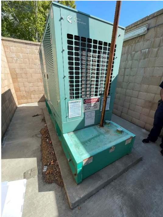
Photograph 42. Backup diesel generator for the Mall at Northgate, located in the parking lot south of Macy's.
