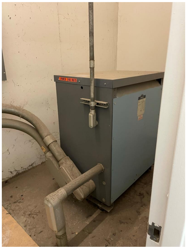
Photograph 22. Transformer in former Sears basement.
