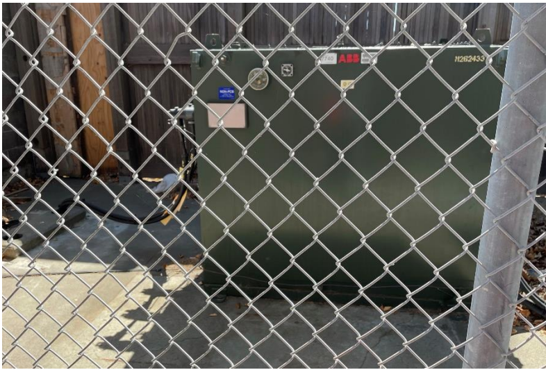
Photograph 27. Macy's transformer in outside wooden in closure.
