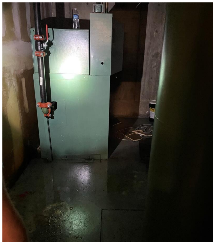
Photograph 18. Passenger elevator equipment room, former Sears basement.
