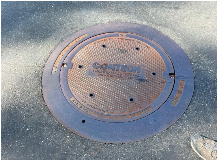
Photograph 41. Hydrodynamic separator in parking lot south of Homegoods.
