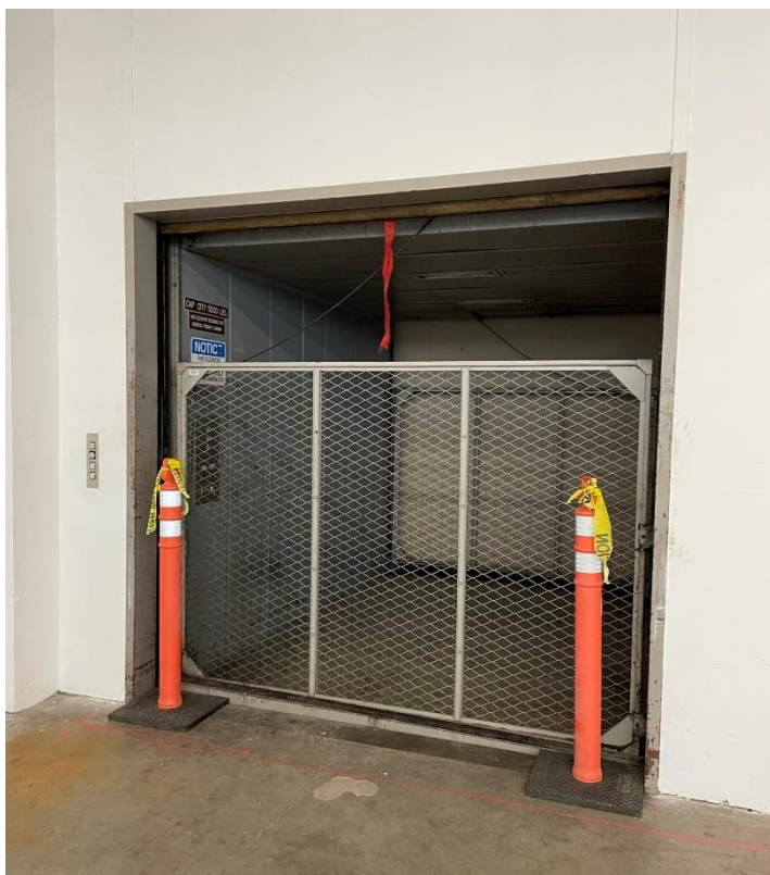
Photograph 17. North freight elevator, former Sears basement.
