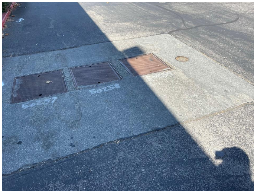
Photograph 2. Clarifier or oil/water separator at north side of auto center building.
