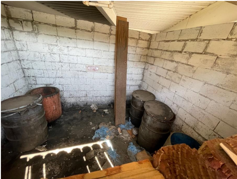
Photograph 43. Grease storage enclosure under the parking structure.
