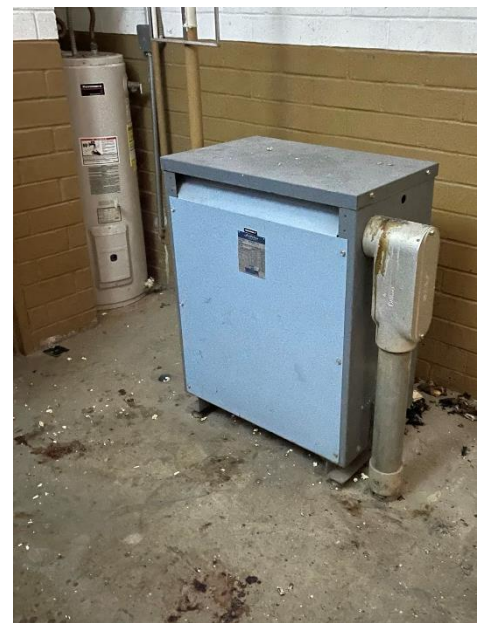
Photograph 13. (Right) Transformer and water heater inside former appliance service building.
