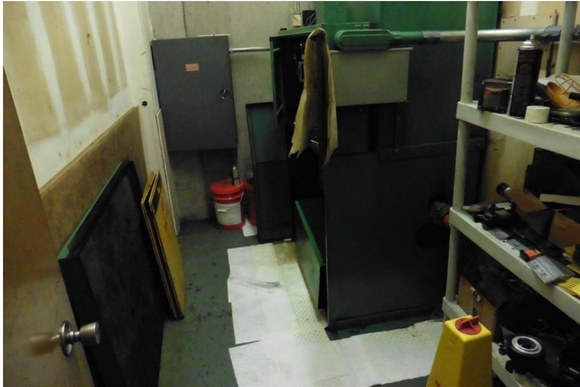
Photo 11: Elevator motor room in Sear's department store basement. Note absorb towels for leaking hydraulic fluid.
