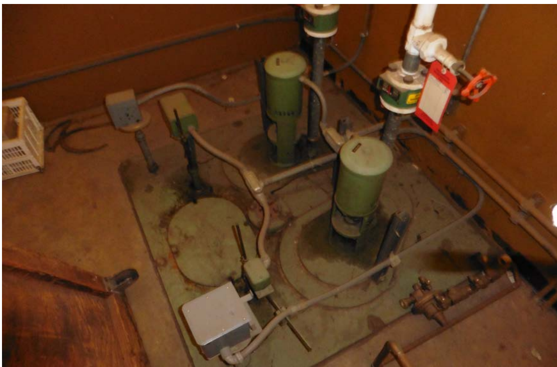
Photo 17: Groundwater pumping system in Sear's basement.
