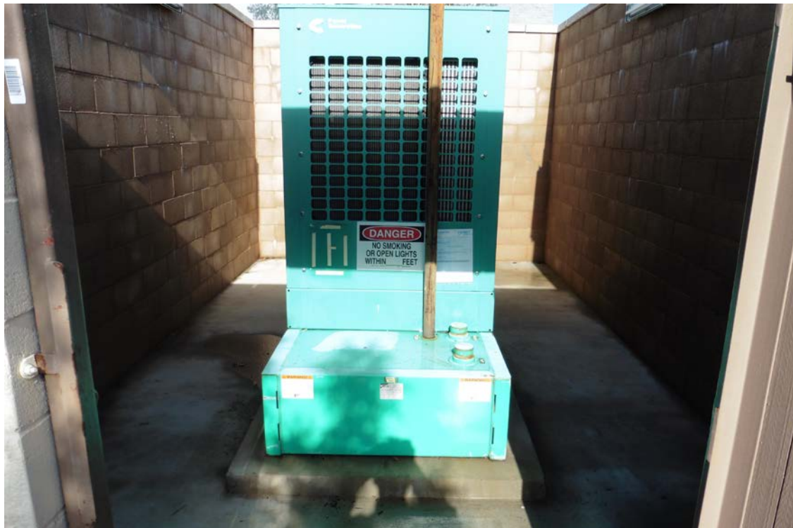
Photo 10: Emergency generator housed in east parking area of Northgate Mall property.
