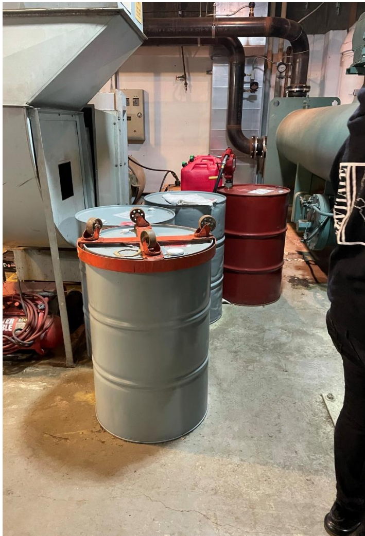
Photograph 25. Macy's backup generator and diesel fuel storage on third floor.
