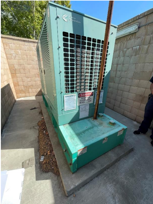
Photograph 42. Backup diesel generator for the Mall at Northgate, located in the parking lot south of Macy's.
