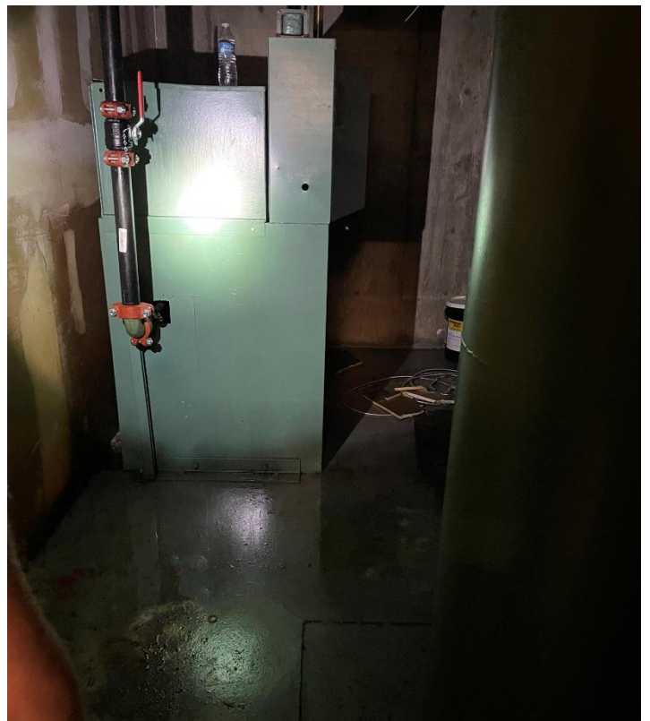
Photograph 18. Passenger elevator equipment room, former Sears basement.
