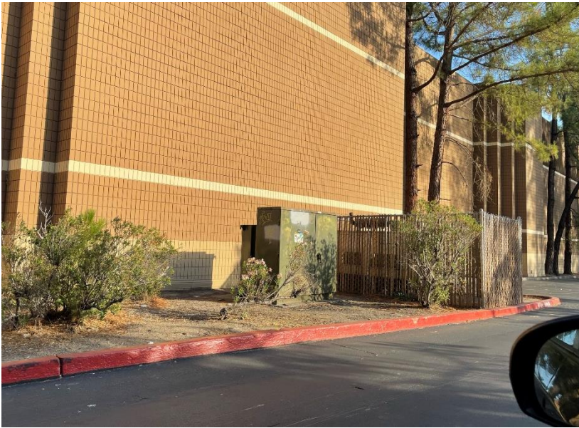
Photograph 33. Kohl's transformer and backup generator enclosure.
