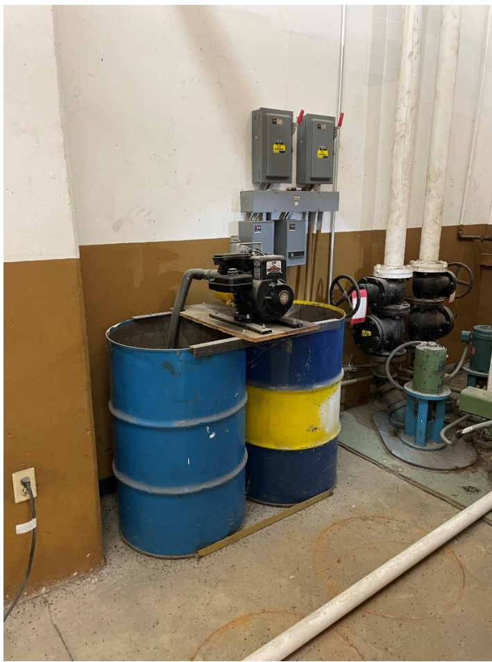
Photograph 21. Drums and sewer, former Sears basement.
