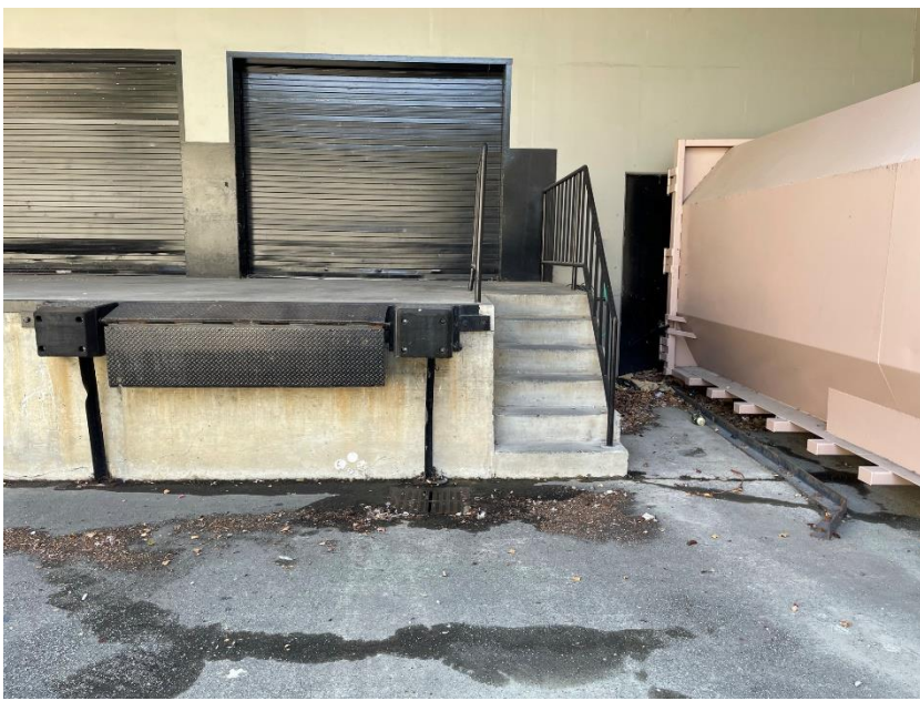
Photograph 14. RH Outlet/former Sears loading dock with trash compactor and storm drain catch basin.
