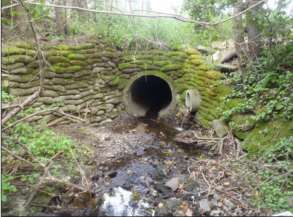
Photo 2. Modern culvert routing Las Gallinas Creek under Los Gamos Drive, view southeast
