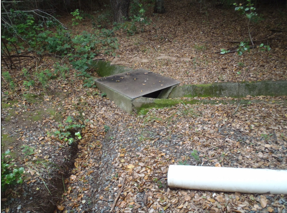
Photo 4. Modern concrete water runoff ditch intersection/angle point with newer dirt ditch with PVC at the bottom of the frame, view southeast
