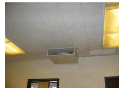
Yellowing, aged fluorescent fixtures and a modified diffuser at City Hall.
