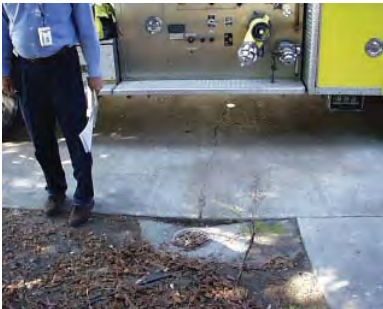
Fire Station No. 7 suffers from drainage problems.
