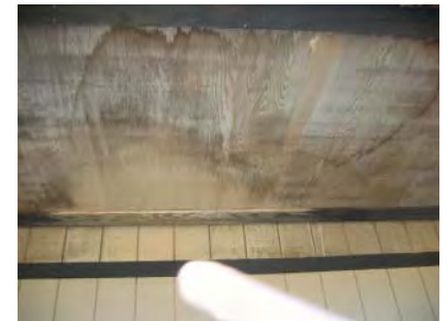
Exterior soffits at San Rafael Community Center show signs of water damage.
