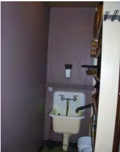
Fire Station No. 4 lacks appropriate space for decontamination
