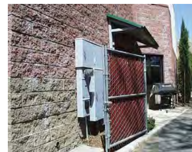
Electrical panels are close to the driveway on Fire Station No. 6's restrictive site.
