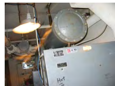
The boiler at City Hall is over 35 years old and past its useful life.
