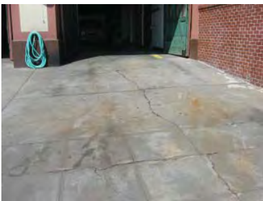
The driveway at Fire Station No. 1 is aged and cracking.
