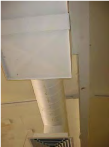
Worn finishes and signs of water leakage in the multipurpose room of Terra Linda Community Center.
