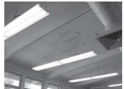
Peeling and staining at ceiling indicate leaking roof
