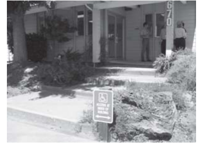
Poor wheelchair access
