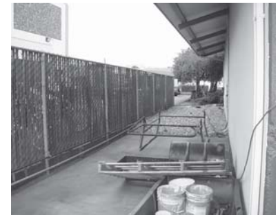
Landscape slopes toward the building on the west side
