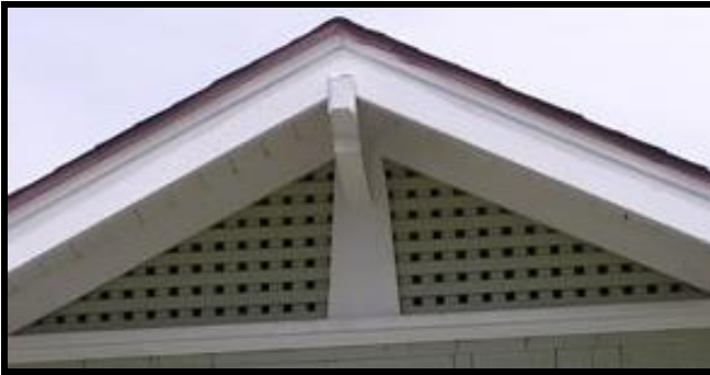
Bungalow Attic Vent
