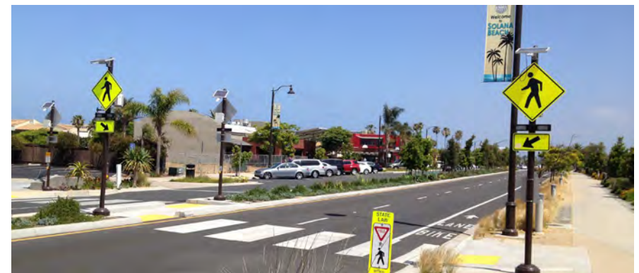
Rectangular Rapid Flashing Beacon (RRFB)
