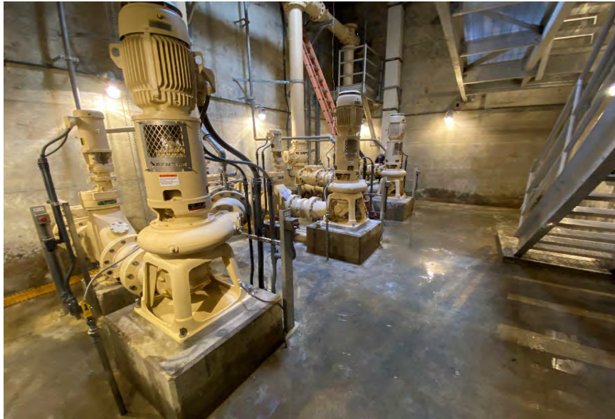
San Lorenzo Sewer Lift Station
