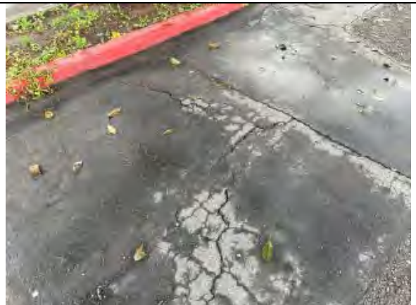
12. Typical cracked asphalt located on Subject Property
