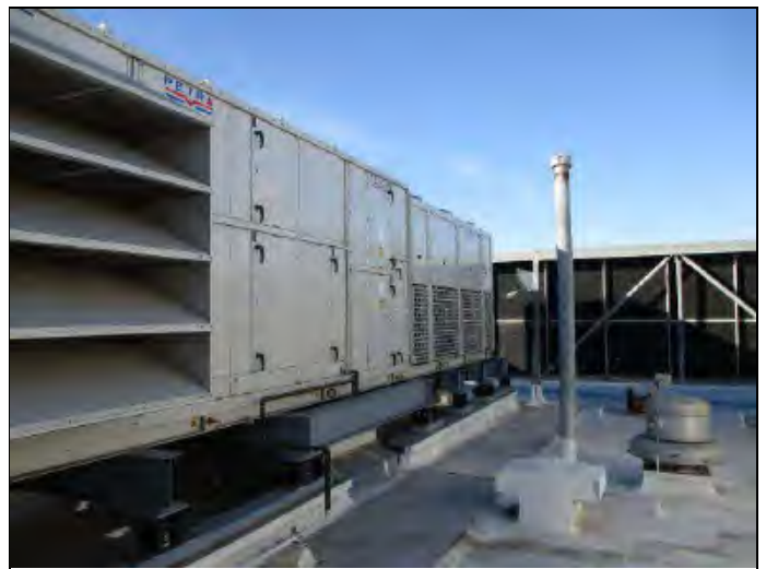
18. Typical "box car" HVAC unit
