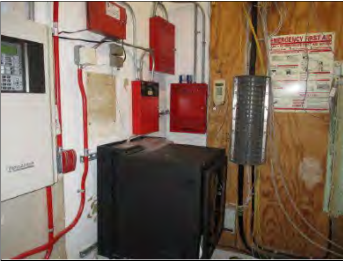
7. Fire alarm control panel
