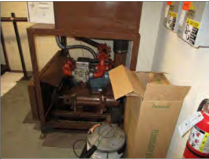
9. Typical elevator equipment
