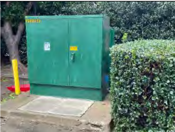
11. Oil-filled transformer located on western portion of Subject Property
