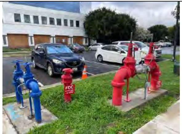
6. Fire connection on northern portion of Subject Property
