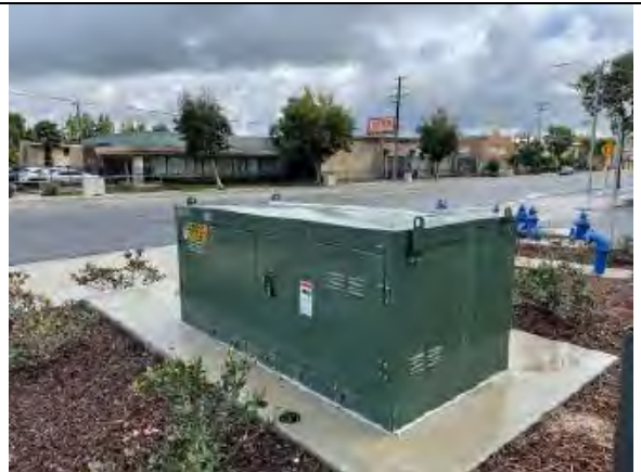
10. Oil-filled transformer located on adjoining property
