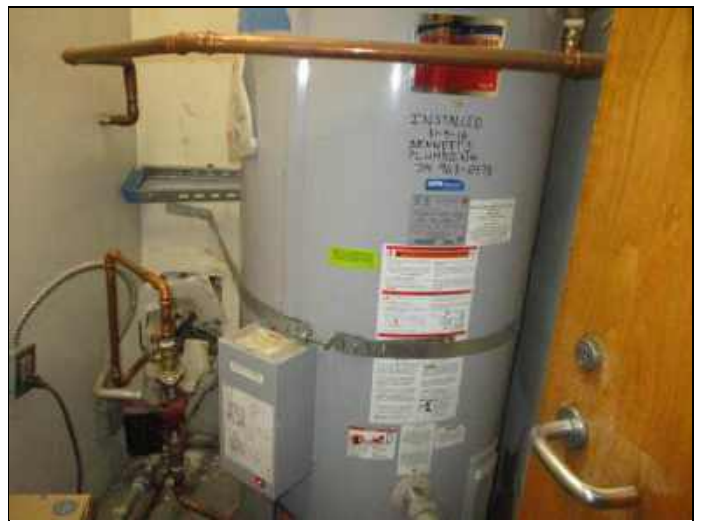
12. Typical gas-fired water heater
