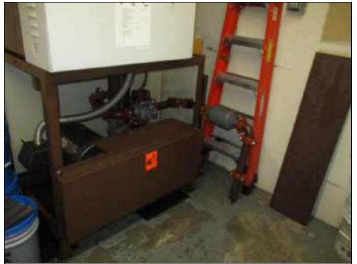
10. Typical elevator equipment
