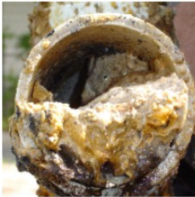
FOG Blockage in Pipe
