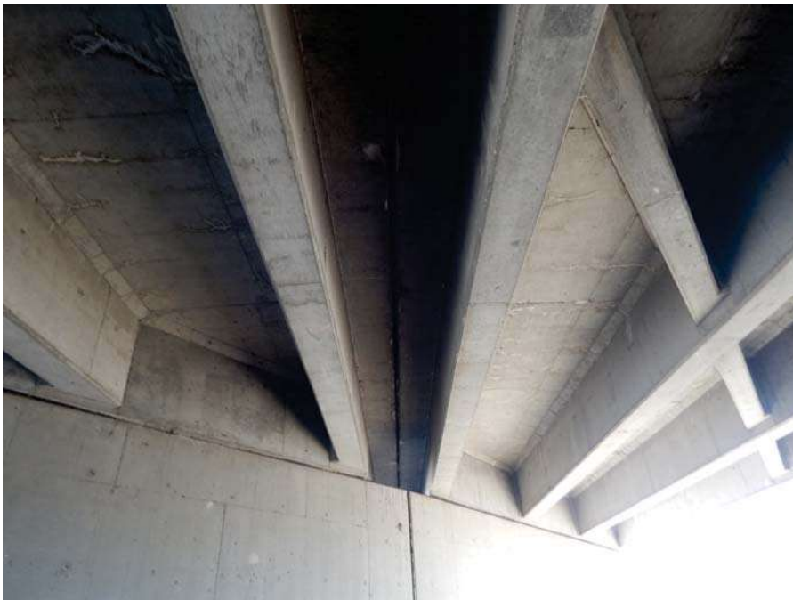
Potentially suitable bat roosting habitat along a hinge in the existing Fairview Street Bridge.
