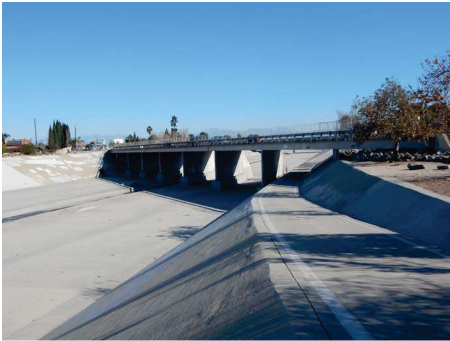
View of the existing Fairview Street Bridge from the Santa Ana River Trail to the west of the bridge, facing east.
