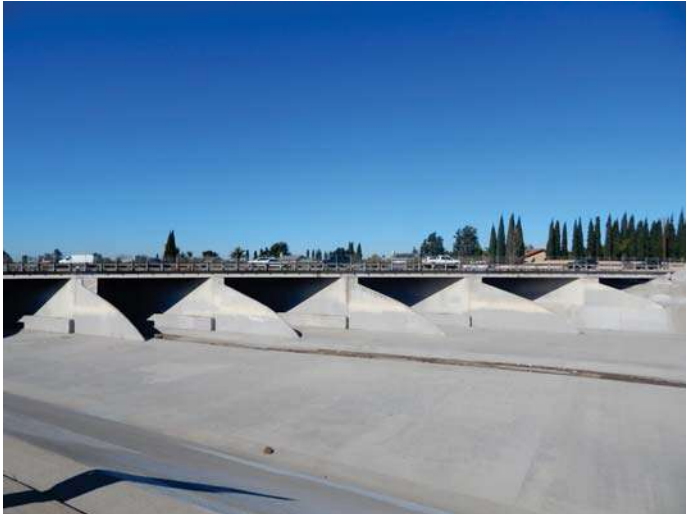
Southwest view, looking at the concrete pier walls of the Fairview Bridge.
