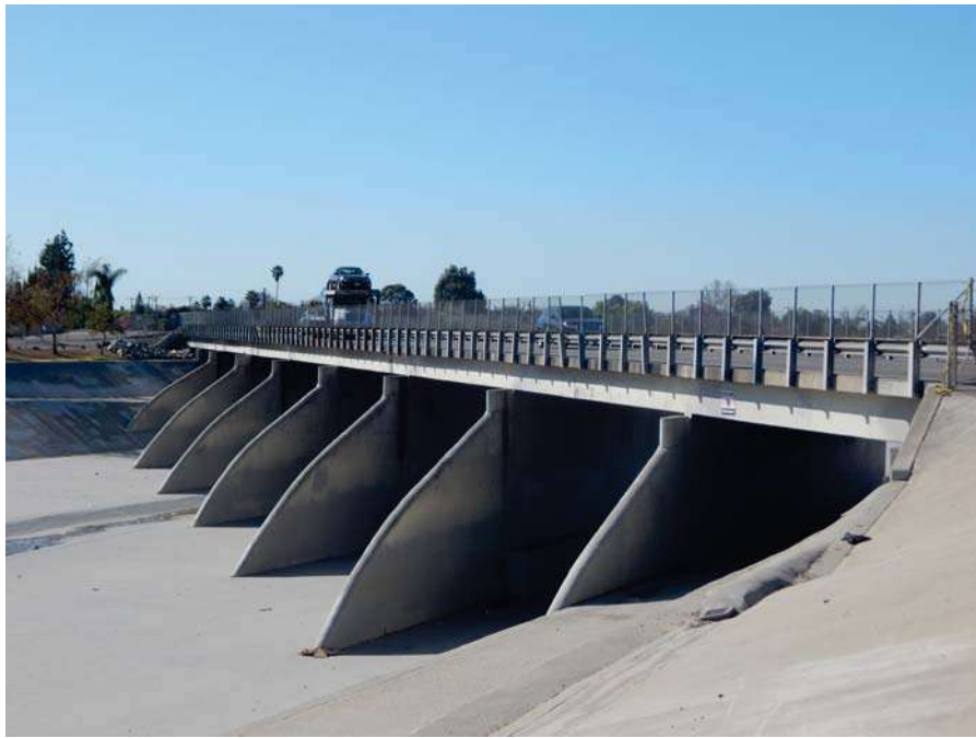
View of the existing Fairview Street Bridge from the top of the north bank of the Santa Ana River channel, facing southwest.
