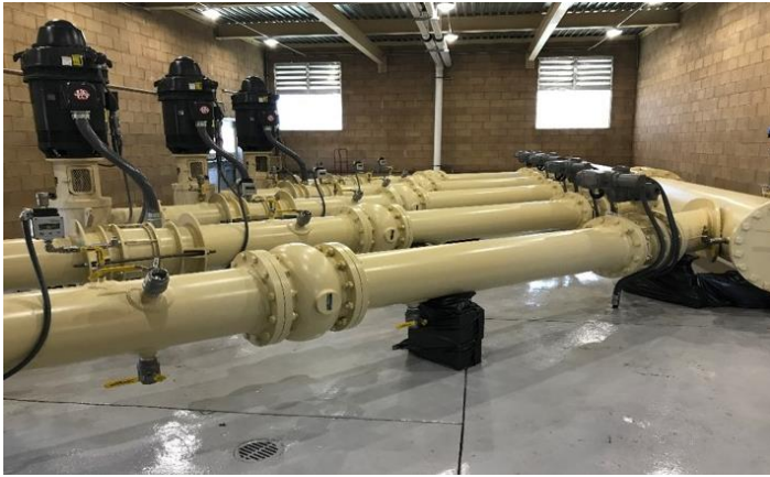
Walnut Pump Station
