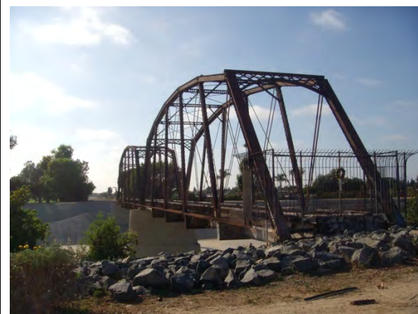
4. Santa Ana River Bridge looking northwest from adjacent Santa Ana River Trail.
