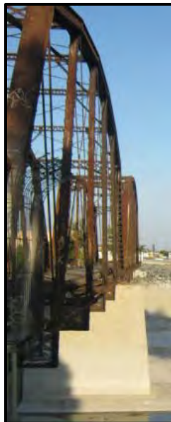
Detail of interior and exterior truss and riverbed pier. View looking East.
