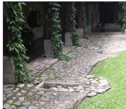
Water retention and control
