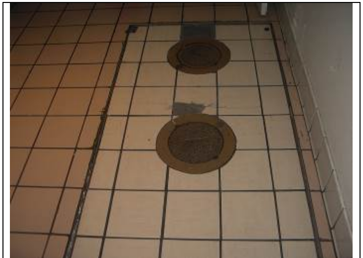
18. View of a grease trap at the subject property.
