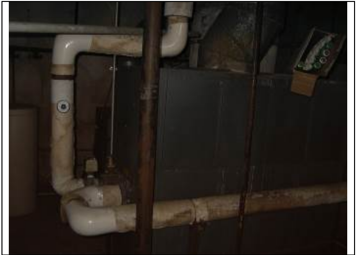
20. View of HVAC room at the subject property.
