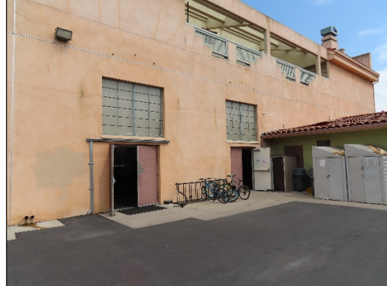
View southeast of the west façade of the two-story/north-south wing. Note the 1980s addition.
