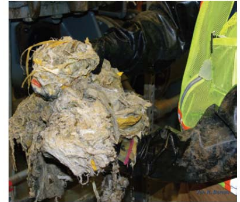
Maintenance crew removing wipes from clogged pumps.
