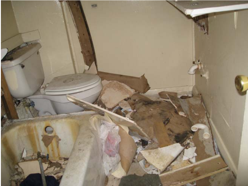
View of debris and the damage caused by transients inside Property structures.
