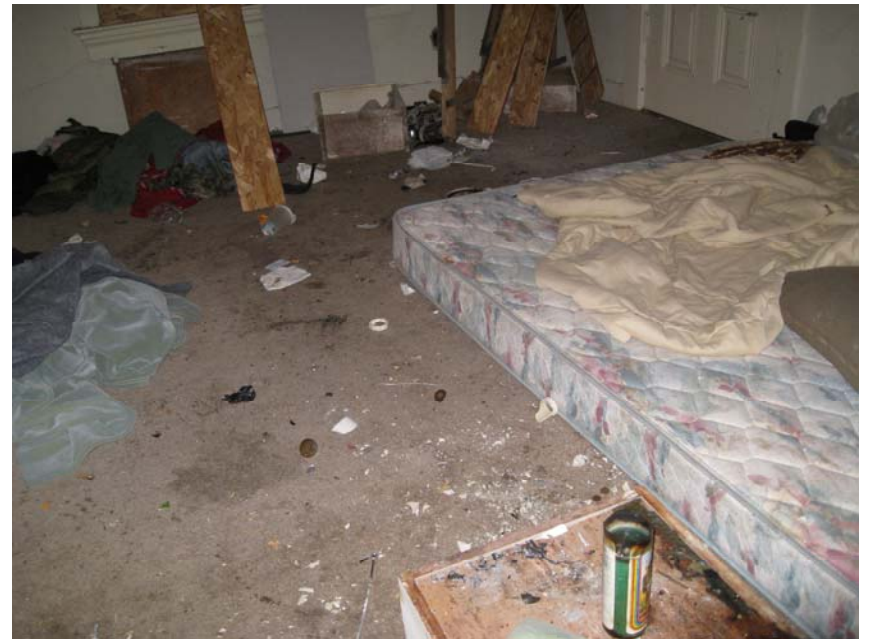
View of debris and the damage caused by transients inside Property structures.
