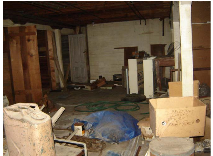
View of storage or debris observed in the basement of 601-603 East 5 th Street.
