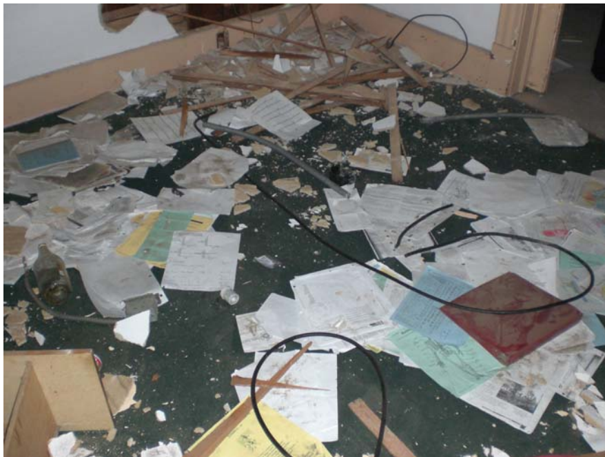
Picture 6: View of household trash and debris inside the 720 E. 6 th Street main building.
