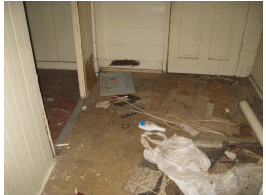
View of debris observed inside the duplexes.
