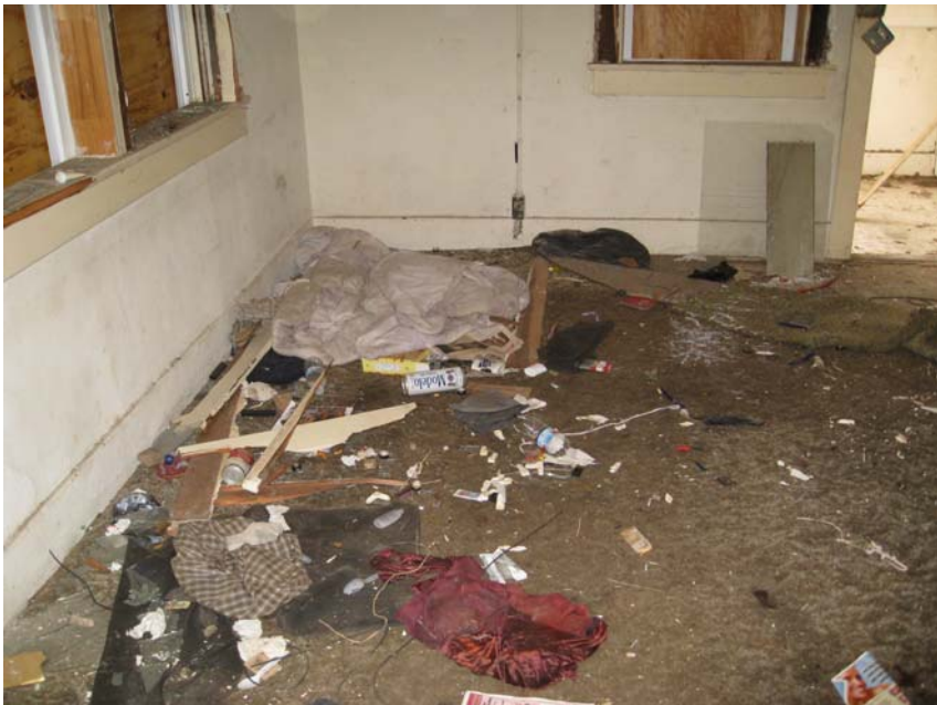
View of debris observed inside the duplexes.
