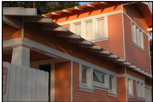
Figure 13-28: Eaves, fascias and soffits should preserve their original characteristics such as rafter tails
