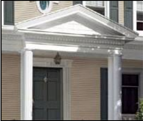
Figure 6-31: Example of Vinyl Siding
