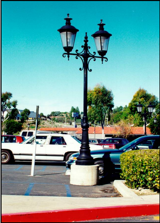
Figure 9-48: Raised bases in parking lots protect from vehicle damage
