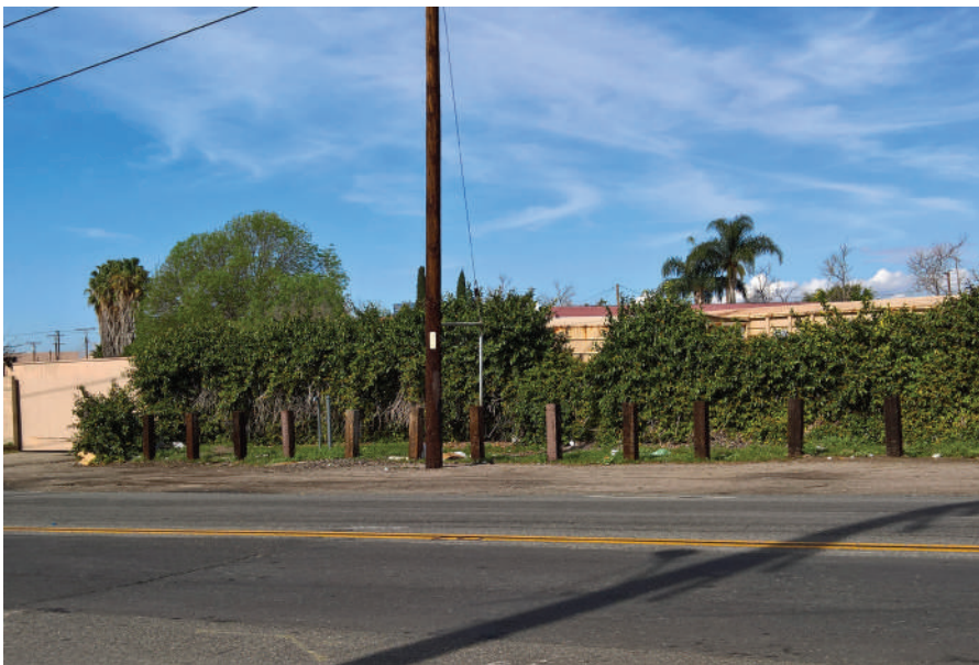
Missing sidewalk and excess right of way
