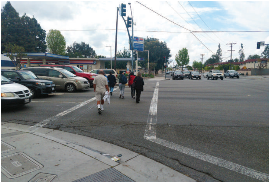
Lack of enhanced crosswalks
