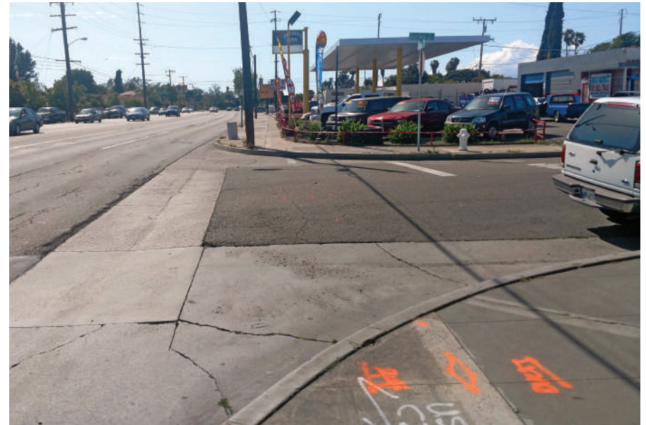
Missing curb ramps
