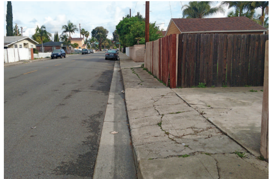
Narrow sidewalks and in need of repair, lack of parkways and street trees
