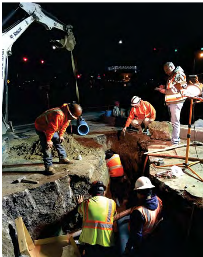
▲ Maintaining utility systems 24-7 [cover photo]
