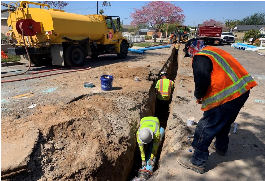
Grovemont Water Main
