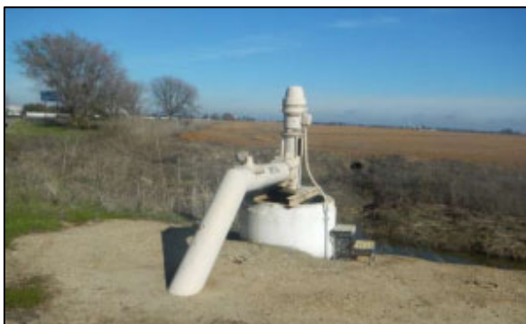
McCune Creek Drain Recovery Pump
