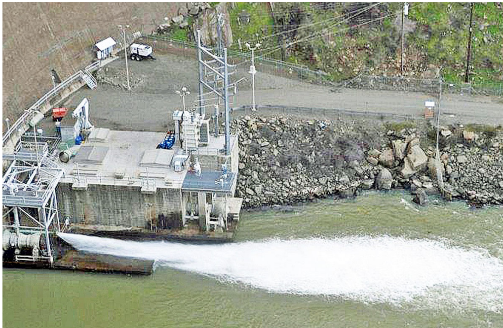
Figure 2-5 SID Power SID Generation Plant at Monticello Dam
