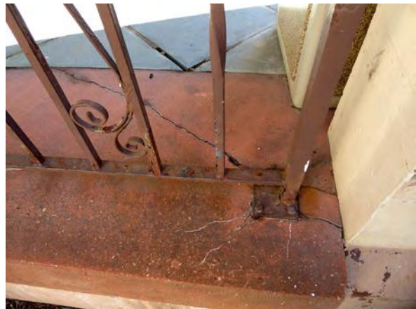
Photo 47: Star cracks caused by rusting rail posts.
