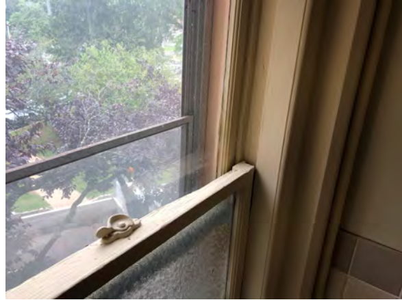
Photo 248: Window on south wall in room 210. Meeting rails do not line up.
