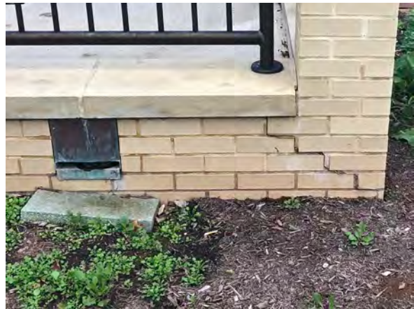
Photo 74: Step crack at base of ramp post (right) and poorly designed drainage of ramp (left).
