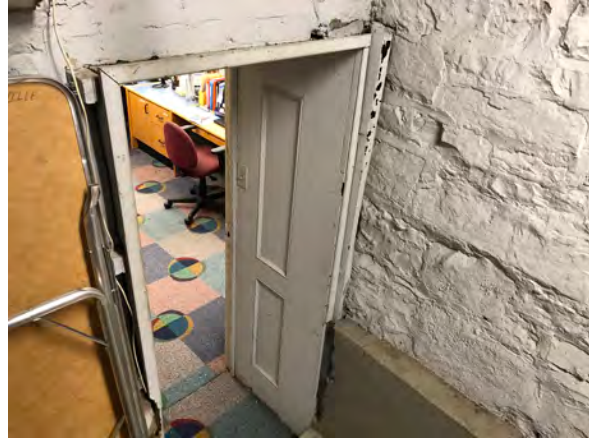
Photo 53: Paneled door jamb on doorway to Room 015 and concrete underpinning under north foundation wall.
