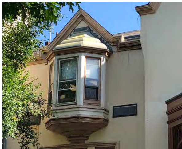
Photo 93: Deteriorated bay window with rolled copper roof on south elevation of Borough Hall.
