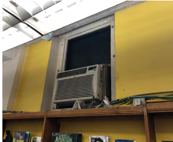
Photo 67: Window air conditioning unit on north wall in Room 015.
