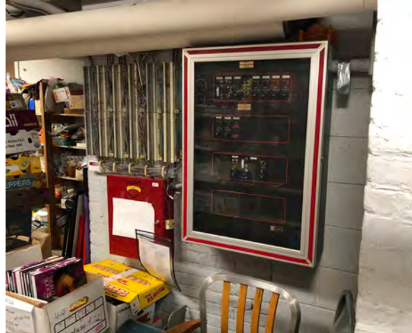
Photo 55: Fire alarm service panel on the south wall in Room 013.
