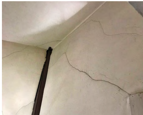
Photo 259: Cracks on wall at third level of northeast stair tower.
