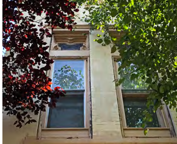
Photo 95: Deteriorated second floor windows with stained glass transoms at south tower.
