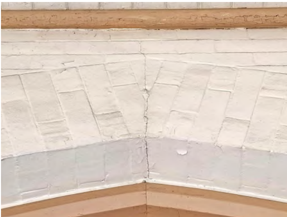
Photo 34: Small crack above main entry door.
