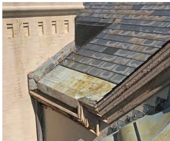
Photo 6: Black sheet membrane behind south tower. Deteriorated flashing on tower and oriel window roof. Slate shingles offset from edge of roof.
