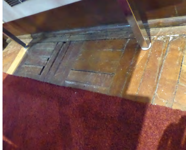
Photo 96: Shrunken boards in southwest corner of Room 100.
