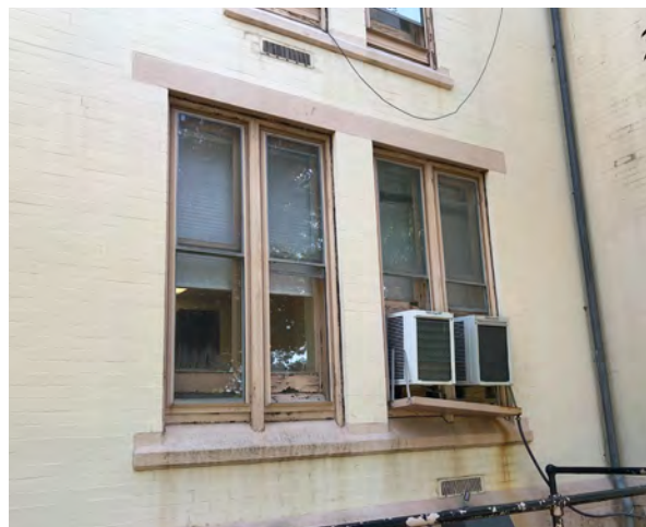
Photo 94: Deteriorated windows at west end of south elevation of Borough Hall.
