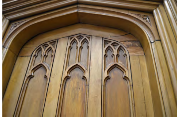
Photo 125: Cracks and area of loss on top wood veneer of door stair tower in Room 103.
