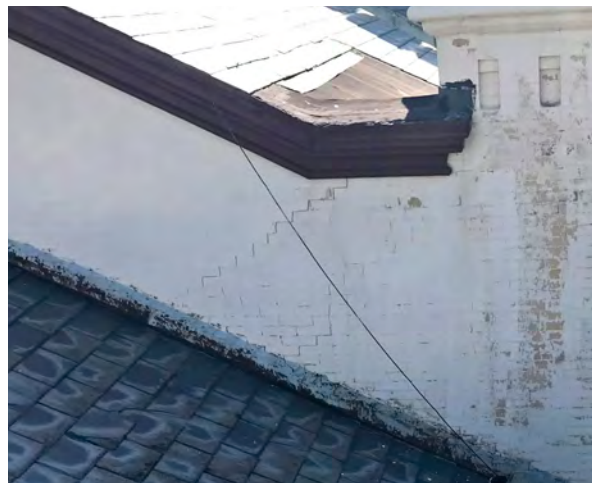
Photo 79: Step cracks and paint loss on west elevation of Borough Hall.
