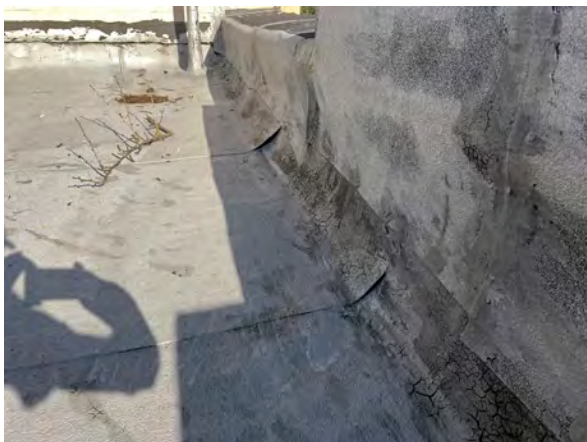
Photo 18: Sheets on Library Addition roof have crazing and are detached along base of parapet.
