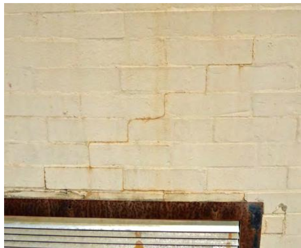
Photo 32: Rusted louver and step crack above on south side of east elevation.
