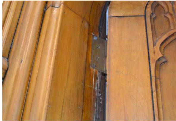
Photo 126: Hinge pulled away from jamb, causing a crack on door to stair tower in Room 103.
