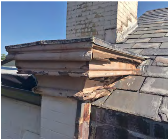
Photo 12: Deteriorated wall dormer step at southwest corner of Borough Hall.
