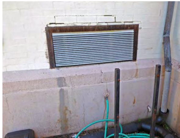
Photo 31: Rusted louver with deteriorated brick above on south side of east elevation.
