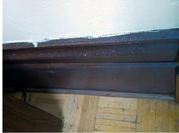
Photo 167: Overpainting and paint flecks on baseboard in Room 112.
