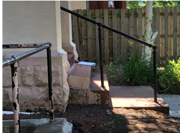
Photo 87: Displaced steps at tower porch.
