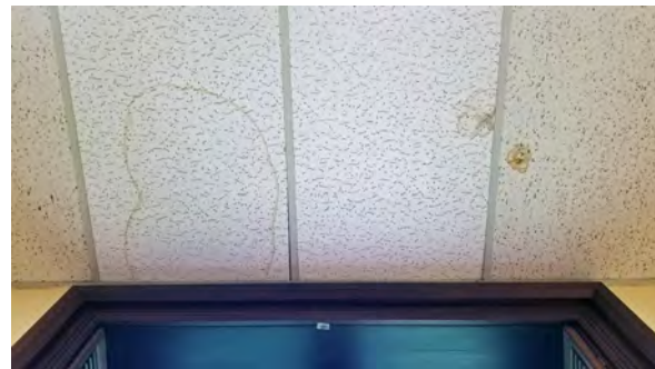
Photo 163: Water stains on drop ceiling tiles at windows of Room 112.
