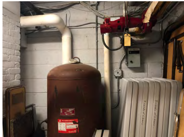
Photo 56: Expansion tank and pump for heating system at east side of Room 013.
