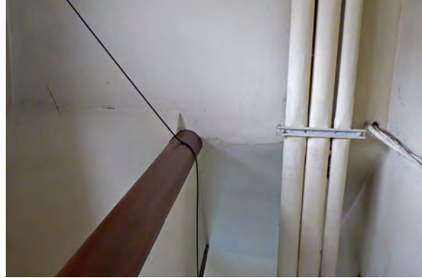
Photo 128: Cracks on ceiling at transition between flat and sloped sections at staircase.
