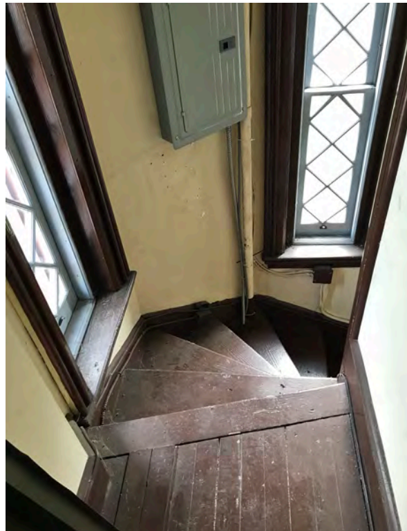
Photo 261: View of landing and spiral stair at third level of northeast stair tower.
