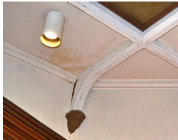
Photo 94: Staining on southwest corner of ceiling in Room 100.
