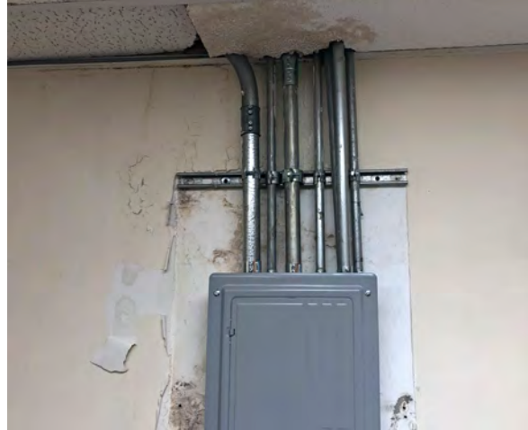
Photo 78: Water damage on north wall and staining on ceiling tile.
