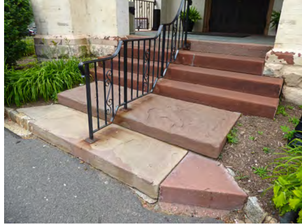
Photo 42: Deteriorated steps to entry porch at east elevation.
