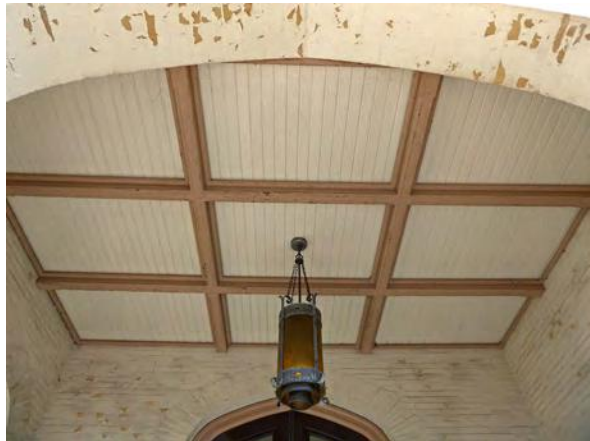
Photo 49: Deteriorated paint on entry porch ceiling.
