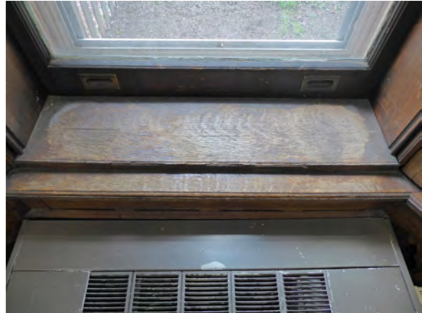
Photo 141: Degraded finish on window sill in Room 104.
