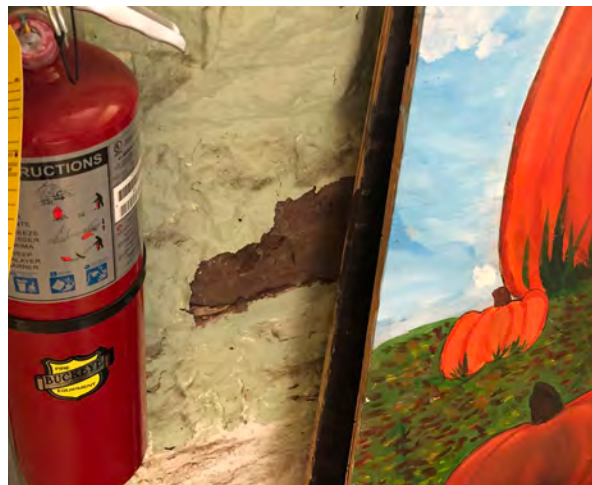
Photo 42: Delaminating stones on south foundation wall.
