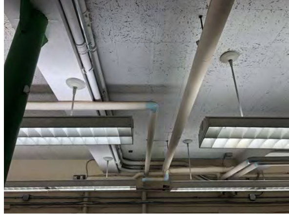
Photo 69: Piping and wiring below applied acoustical ceiling tile in Room 015.
