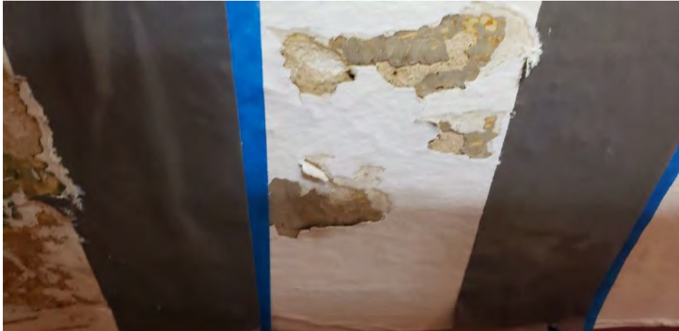
Figure 14. Pre-existing conditions and detachment between paint layers at ceiling level in Room 100; difficulty in installing exposure windows.
