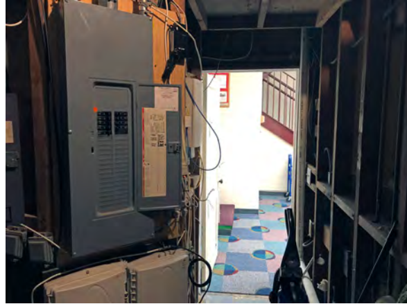
Photo 83: View south in Room 020, showing electrical service equipment at left and unfinished west wall to the right.
