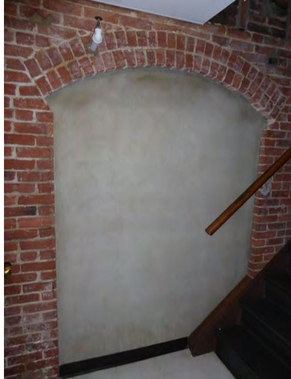
Photo 4: Filled in arched opening in brick interior foundation wall at bottom of basement stairs.
