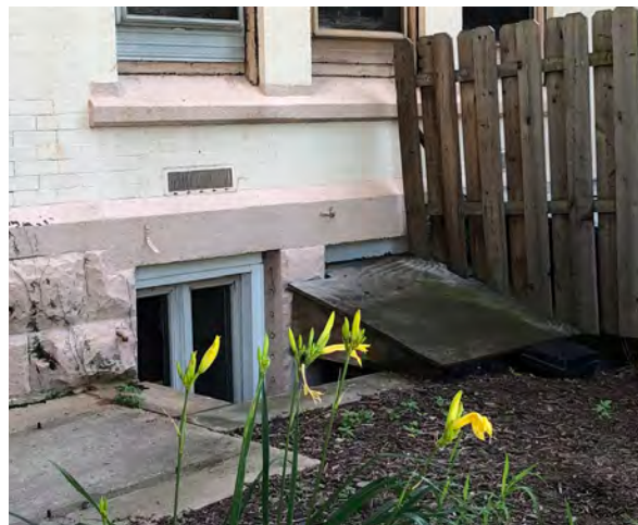
Photo 91: Foundation windows with light wells at east end of south elevation of Borough Hall.
