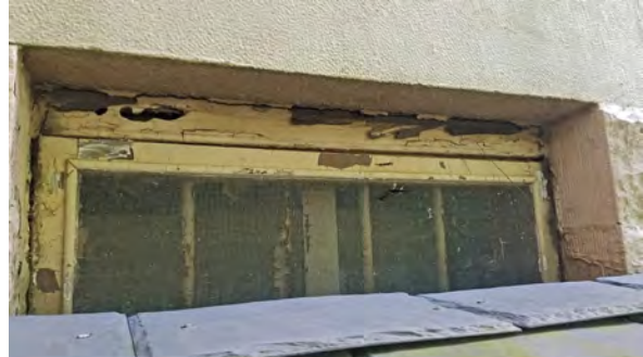
Photo 63: Typical condition of deteriorated foundation windows on north elevation of Borough Hall.
