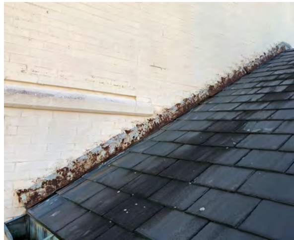
Photo 8: Typical condition of deteriorated flashing along brick walls of Borough Hall.
