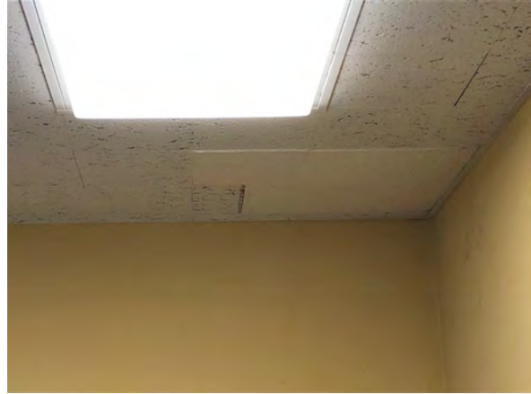
Photo 242: Patched area of acoustical tile ceiling in southeast corner of Room 209.
