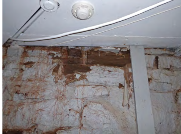
Photo 30: Delaminating stones on south wall in Room OST-2.
