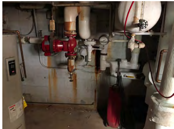
Photo 50: View north in Room 012 showing hot water heater and boiler piping.
