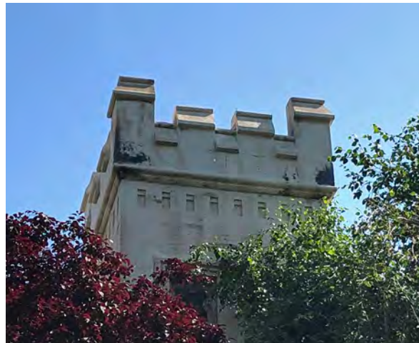
Photo 84: Black deposits, likely manganese oxide, on crenellations of south tower.
