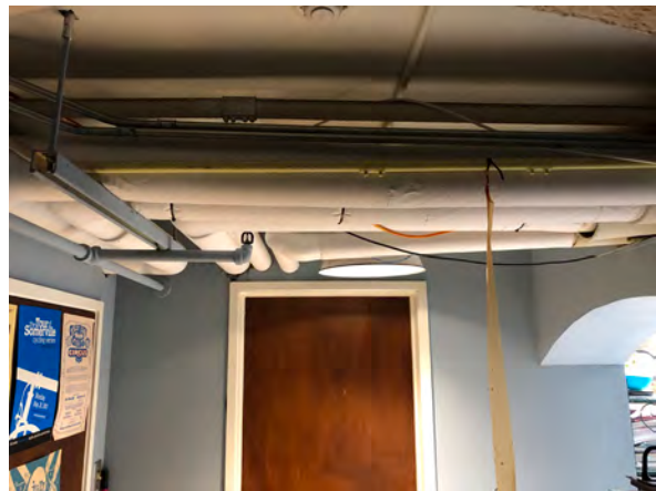
Photo 11: Exposed piping at ceiling outside of closet in Room 002.
