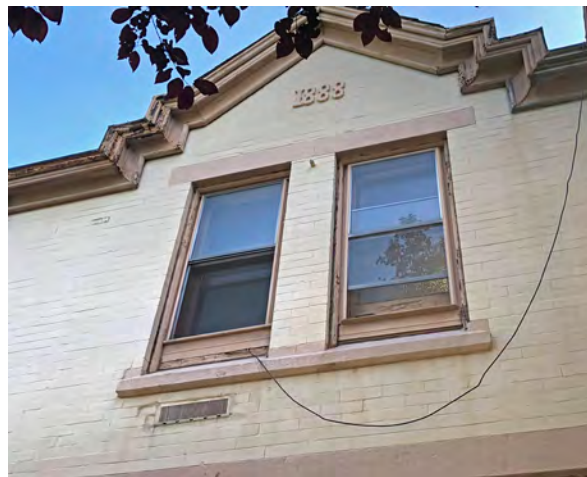
Photo 96: Deteriorated windows at west end of south elevation of Borough Hall.
