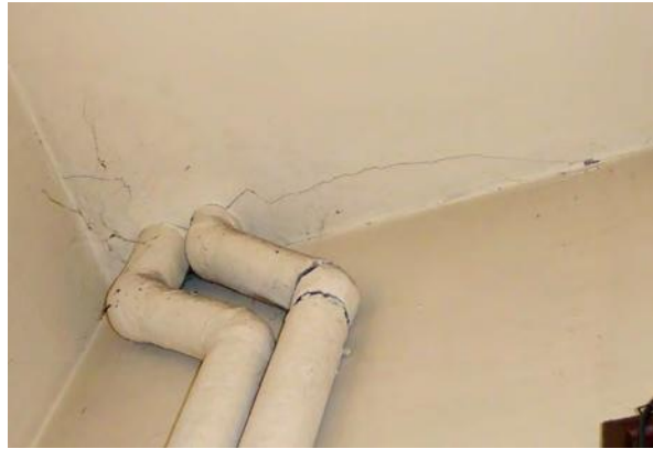
Photo 129: Cracks in ceiling around pipes.
