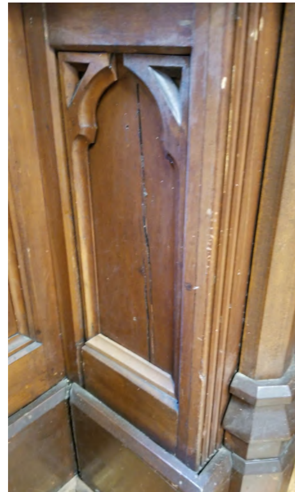
Photo 168: Crack and small loss on wood panel below windows in Room 112.
