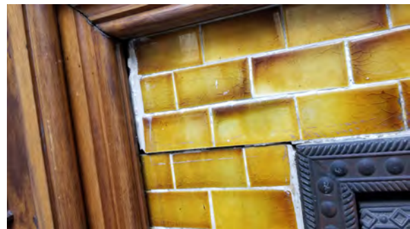
Photo 170: Displaced ceramic tiles on top corner of fireplace surround.
