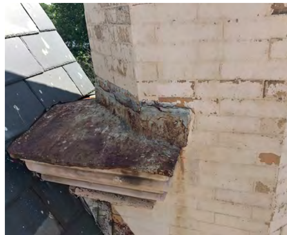
Photo 11: Typical condition of deteriorated flashing capping wall dormer steps on Borough Hall. Taken from south elevation.
