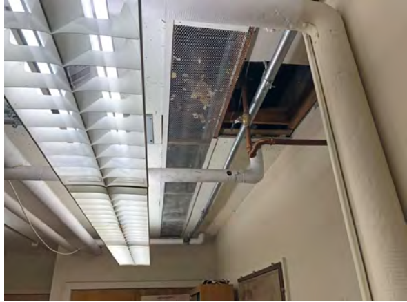
Photo 73: Wire mesh covering section of removed tiles at north end of ceiling. Source of leak at left.
