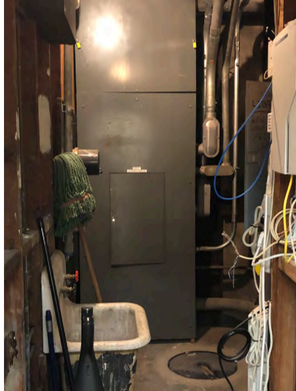
Photo 86: Electrical service equipment throughout, utility sink on west wall and unused sump pump pit on floor in Room 020.
