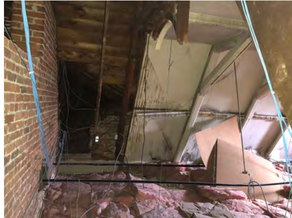
Photo 230: Vaulted ceiling concealed behind dropped ceiling in Room 207. Portion of ceiling lost at left.
