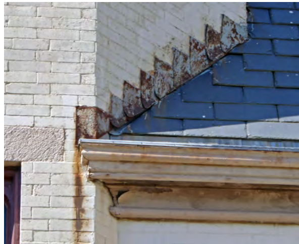
Photo 9: Typical condition of deteriorated flashing along brick walls of Borough Hall.
