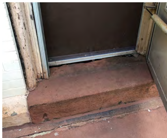
Photo 97: Void at west entry door sill.
