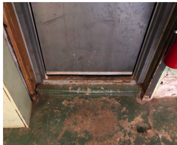
Photo 44: Rust on the exterior door threshold in Room 011.
