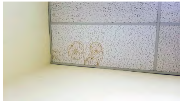
Photo 164: Water stains on drop ceiling tile at southwest corner of Room 112.
