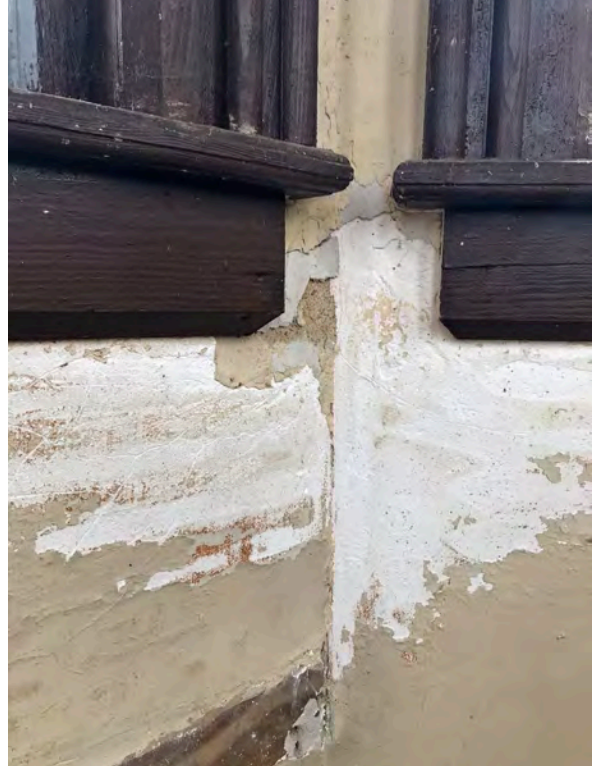
Photo 270: Paint loss on wall in northeast stair tower.
