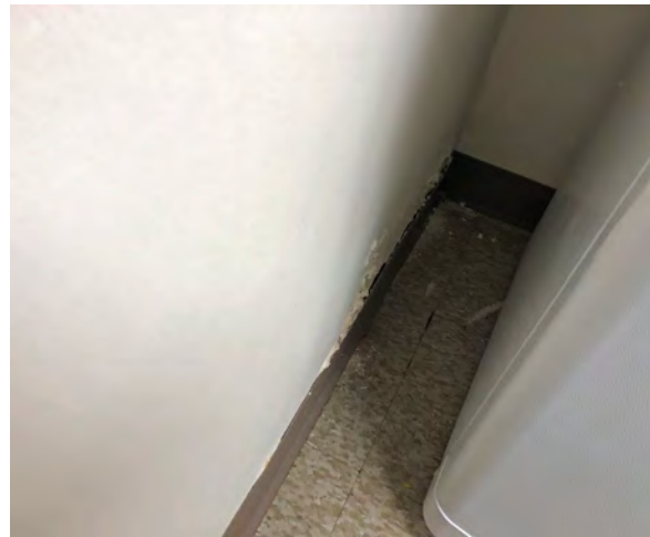
Photo 79: Water damage at bottom east corner of the north wall, by the refrigerator.
