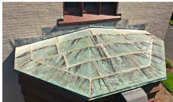
Photo 85: Copper roof on bay at east end of south elevation of Borough Hall.
