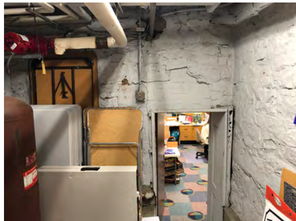
Photo 52: West wall in Room 013 with door to Room 015 and brick repair above.
