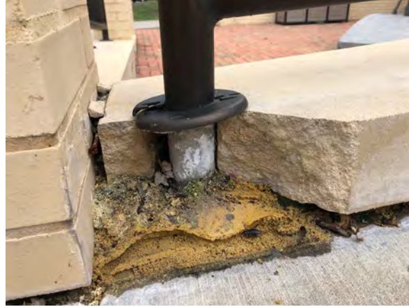
Photo 70: Total loss of portion of ramp coping.
