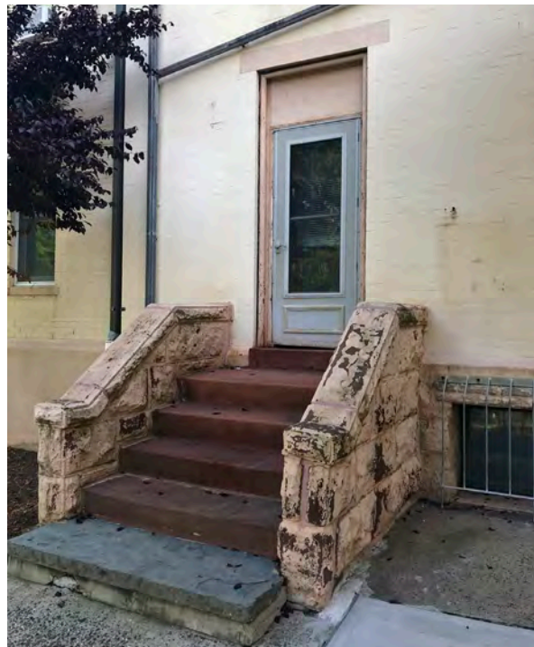
Photo 88: Displaced west steps and sidewalls.
