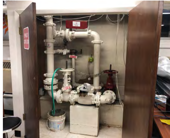
Photo 39: Sprinkler control room on the north wall of Room 010.
