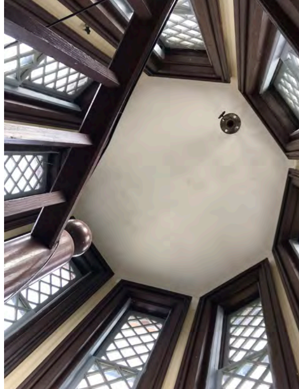
Photo 263: Repaired ceiling of top room in northeast stair tower.
