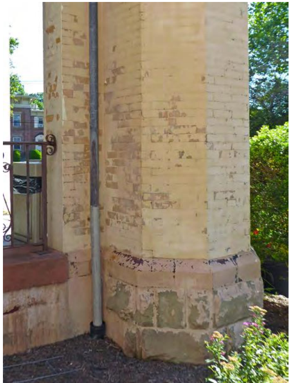
Photo 36: Paint loss at south tower of east elevation.
