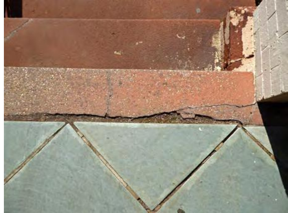
Photo 45: Deteriorated cast stone edging and slate paver joints at entry porch.
