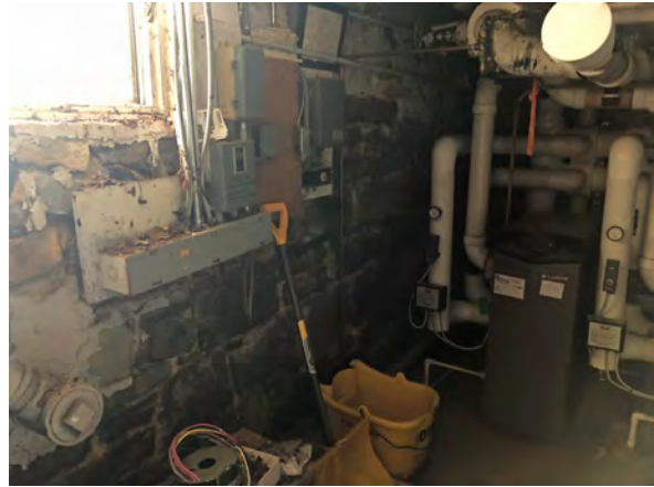
Photo 49: Southeast corner of Room 012 showing one boiler and associated piping.
