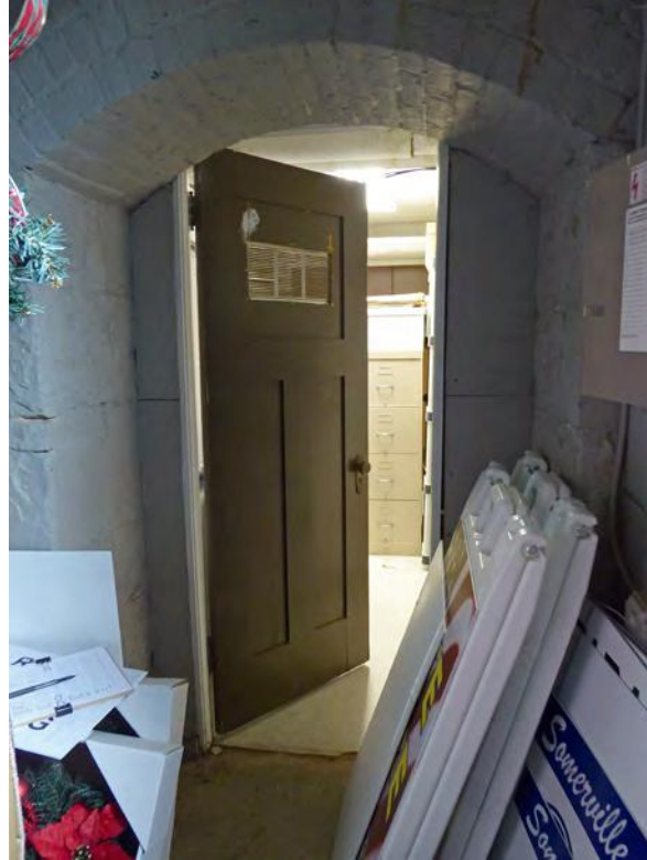
Photo 28: View west in Room OST-2 showing archway in brick foundation wall and door to Room 006.
