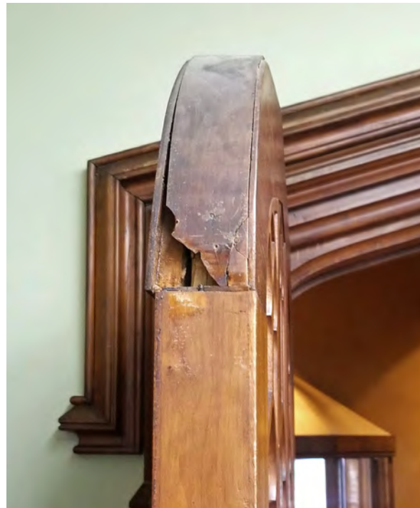
Photo 176: Detached veneer and area of loss at top of door into Room 101.
