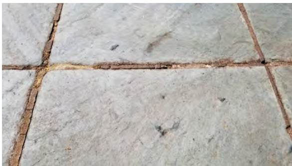
Photo 48: Deteriorated slate paver joints at entry porch floor.
