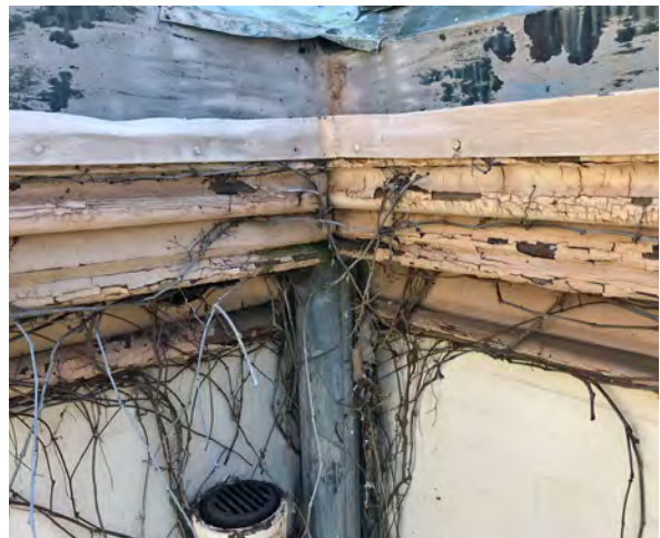
Photo 15: Detail view of deteriorated cornice on Borough Hall.
