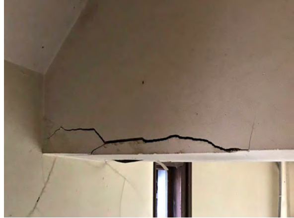
Photo 258: Crack and associated detachment of plaster on beam at third level of northeast stair tower.
