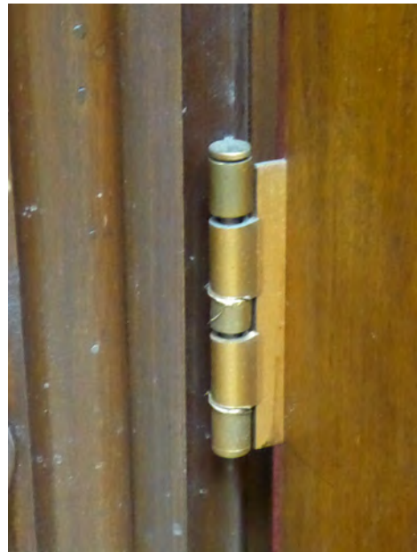
Photo 166: Distressed hinge on the door to Room 101.
