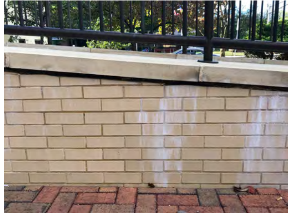
Photo 73: Salt efflorescence on brick wall of ramp.
