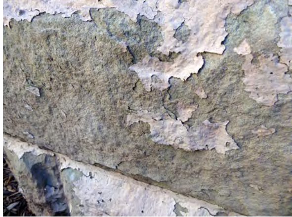
Photo 35: Delamination and subsequent paint loss on foundation stones on east elevation.
