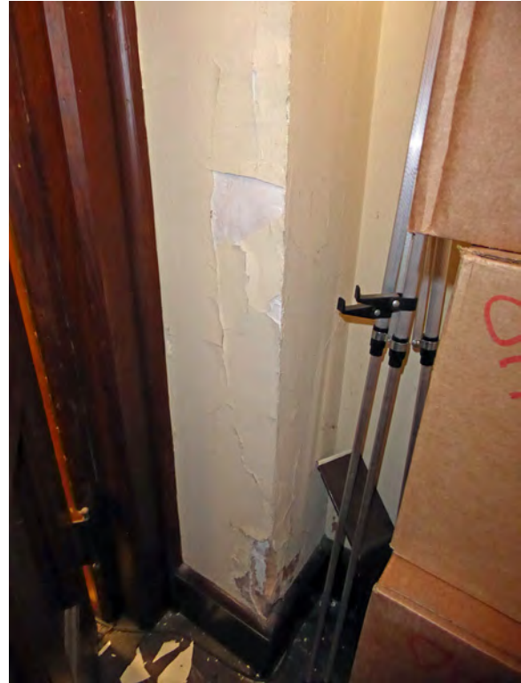
Photo 131: Cracks and areas of loss on wall behind door connecting to Room 103.
