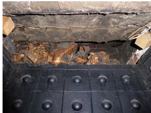
Photo 145: Firebox interior showing open flue, shims under support beam and crack in plaster on beam.
