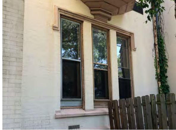
Photo 92: Set of three deteriorated windows at first floor of south elevation of Borough Hall.
