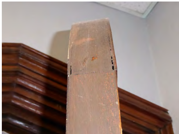
Photo 140: Veneer detached at top of door connecting to Room 115.
