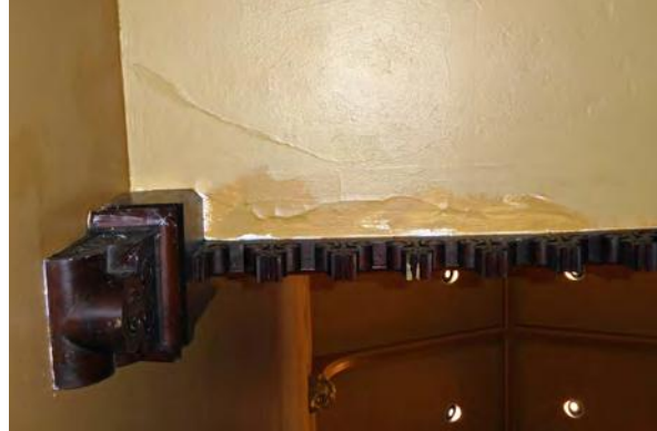
Photo 104: Cracks on ceiling at stair opening in Room 101.
