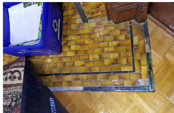
Photo 171: Missing ceramic tiles on fireplace hearth.
