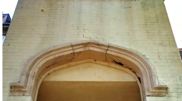
Photo 86: Cracks in stone archway and bricks above at tower porch.
