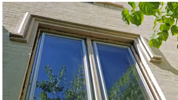
Photo 65: Deteriorated sealant around first floor window N108.
