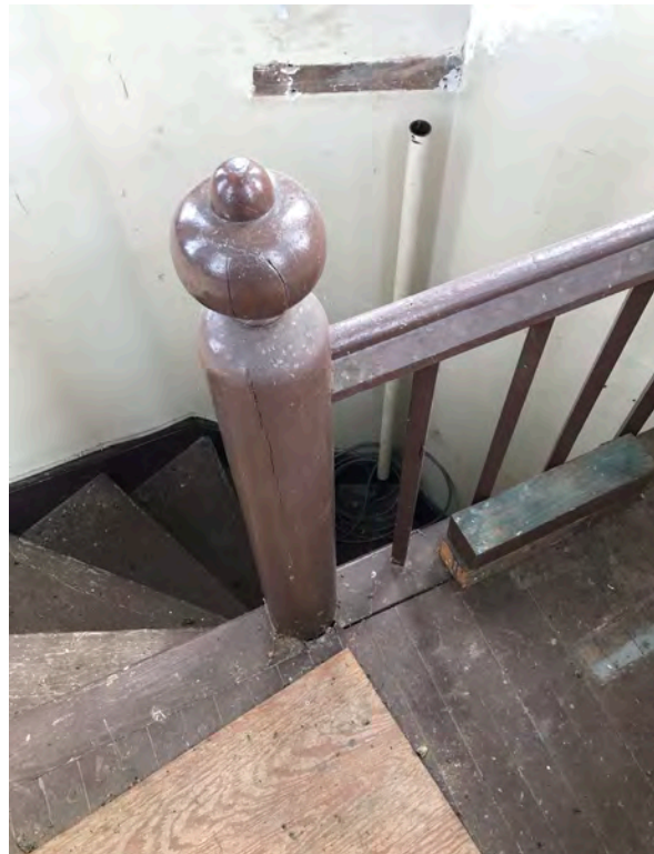
Photo 264: Wood post and guardrail at landing in top room in northeast stair tower.
