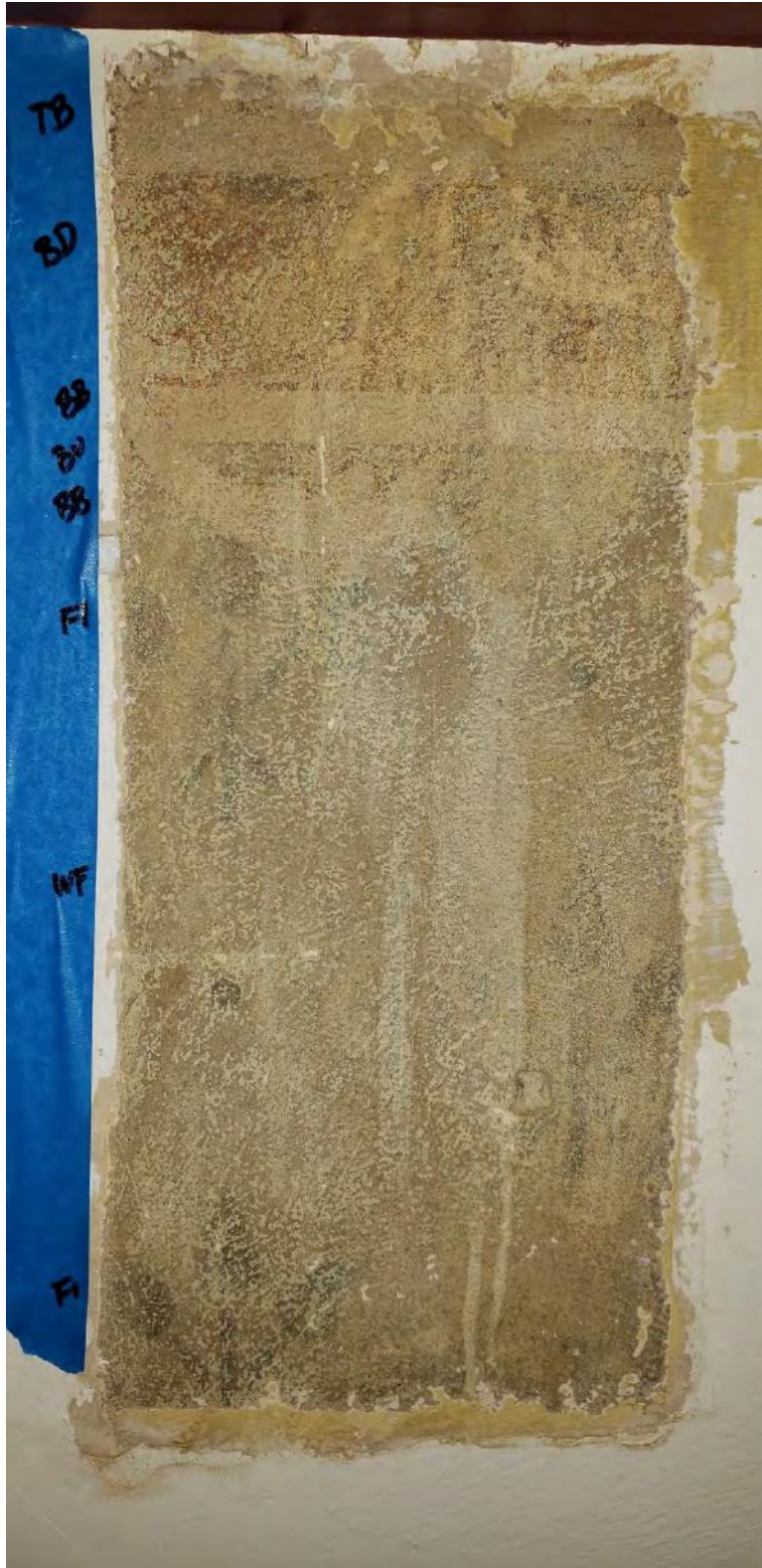
Figure 5. Preliminary exposure window on wall surface in Room 100 indicates presence of ca. 1888 geometric and floral stenciling on a wall surface. Exposure did not indicate presence of early 20 th century ornament, but some ornament or decoration was suggested by cross-section analysis.
