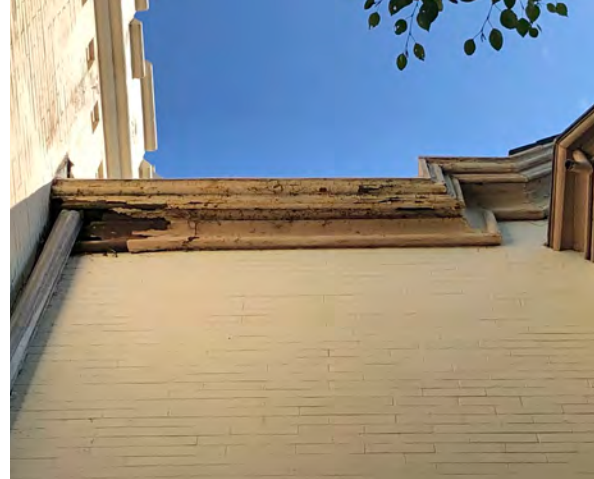
Photo 98: Deteriorated wood cornice at east end of south elevation of Borough Hall.
