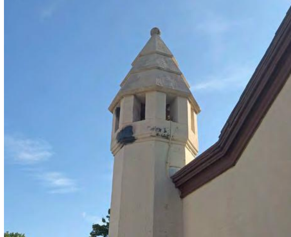
Photo 26: Black deposits, likely manganese oxide, on sandstone cap of northwest chimney.
