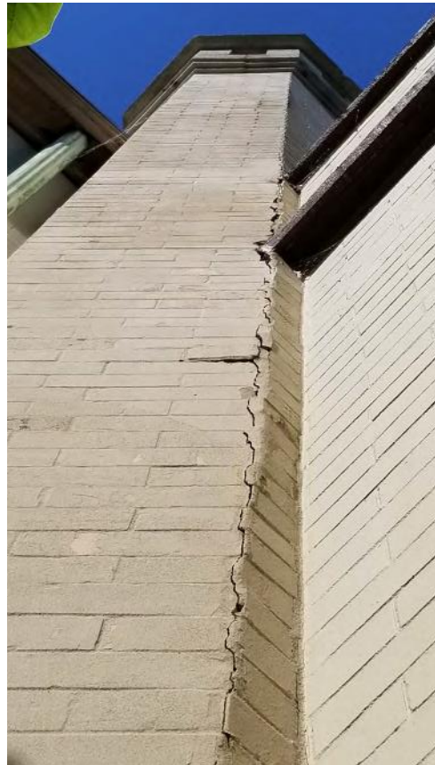
Photo 60: Crack along northwest chimney at intersection with Library addition.
