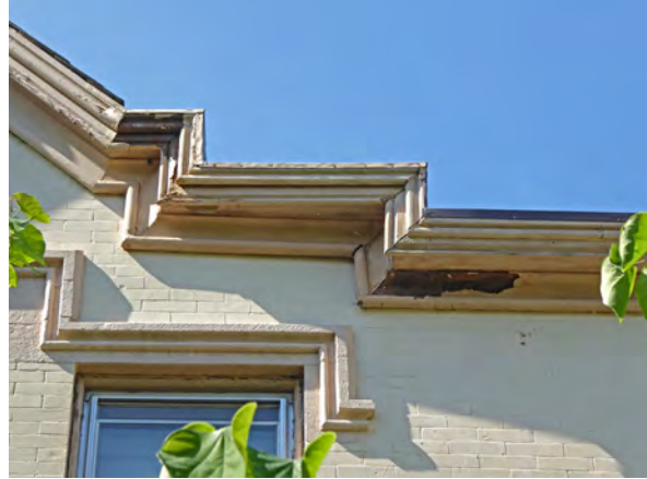
Photo 66: Deteriorated wood cornice at north elevation of Borough Hall.
