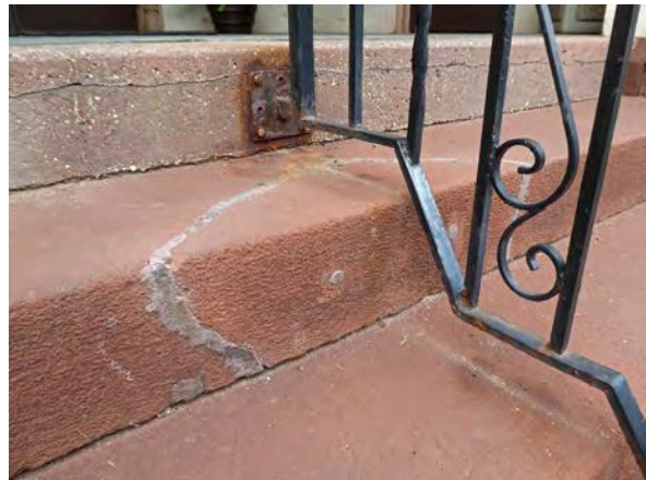
Photo 43: Rusting iron railing and extensive cracking on entry porch steps.
