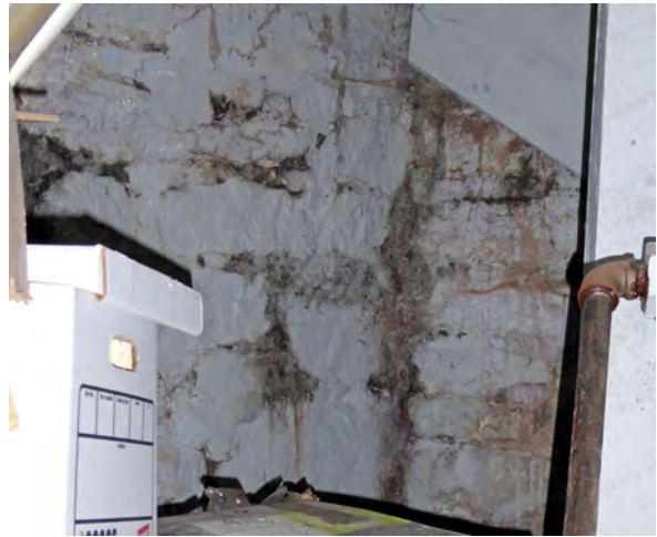
Photo 31: Black mold in the northeast corner of Room OST-2.
