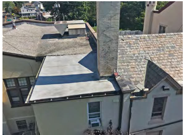
Photo 2: View from the east side of the building of slate roofs on Borough Hall, the sheet membrane roof on the rear addition, and membrane roof with ballast on the Library. Also note the step cracking on the square boiler chimney.
