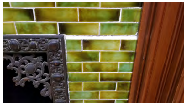
Photo 181: Displaced ceramic tiles on top corner of fireplace surround.
