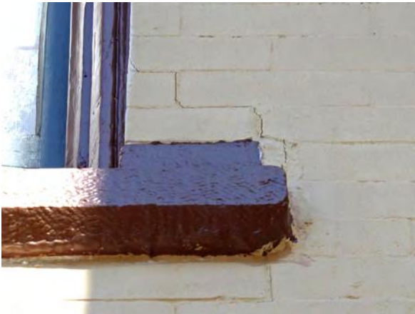
Photo 33: Example photo of cracking around sills on east elevation.
