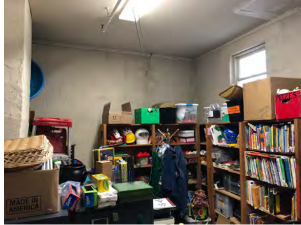
Photo 57: View south in Room 014. Note the water staining at the top of the wall.
