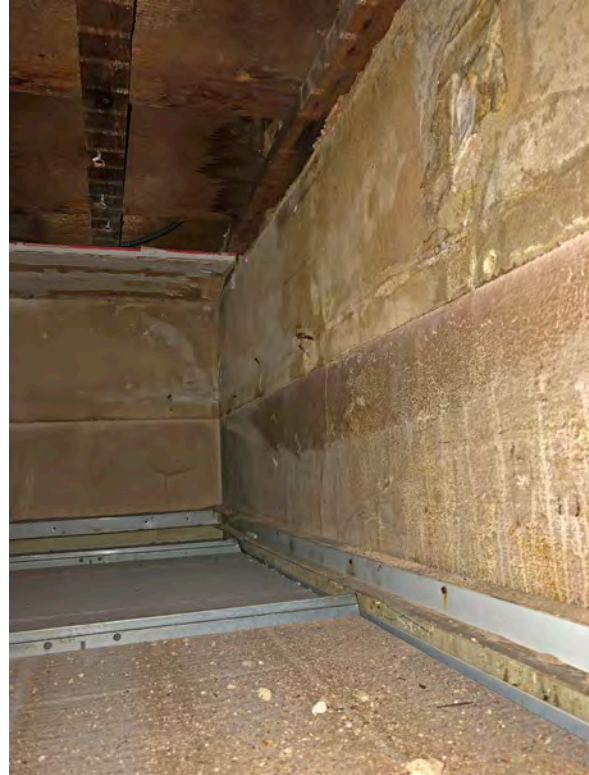
Photo 175: View above drop ceiling showing that historic plaster ceiling has been removed.
