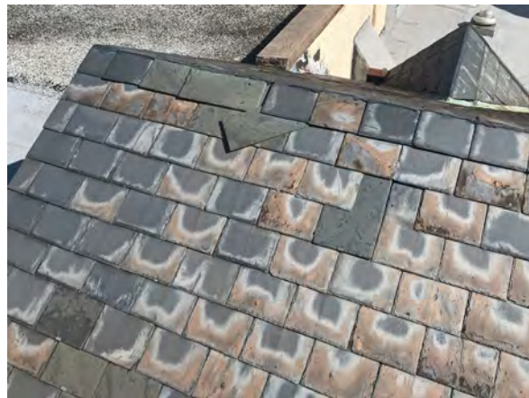
Photo 5: Replacement slates on west roof of Borough Hall. Taken from south elevation.
