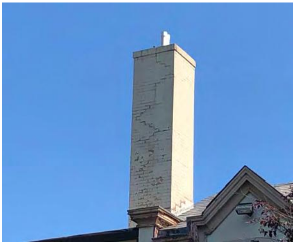
Photo 25: Extensive step cracking on boiler chimney at southwest corner of Borough Hall.
