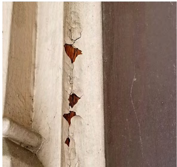
Photo 58: Paint loss at archway around entry door showing possible historic graining beneath.
