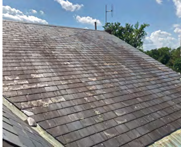
Photo 4: Black algae and lichen growth on west roof of Borough Hall. Taken from north elevation.
