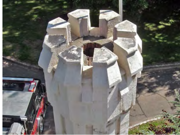
Photo 37: South tower roof with opening and cracked parging.
