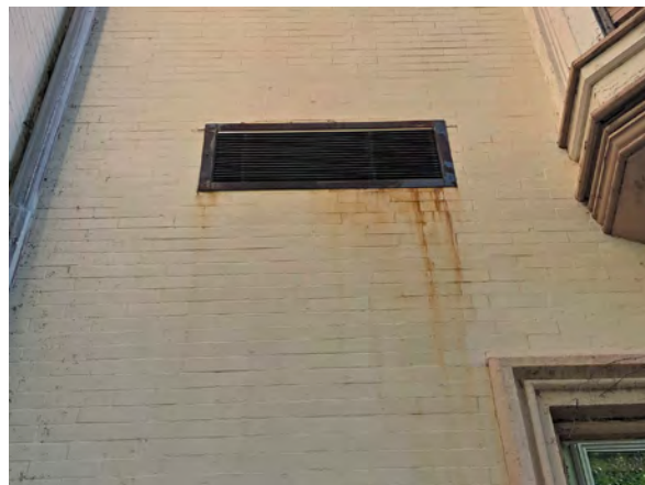
Photo 90: Rusted louver at second floor on east end of south elevation.
