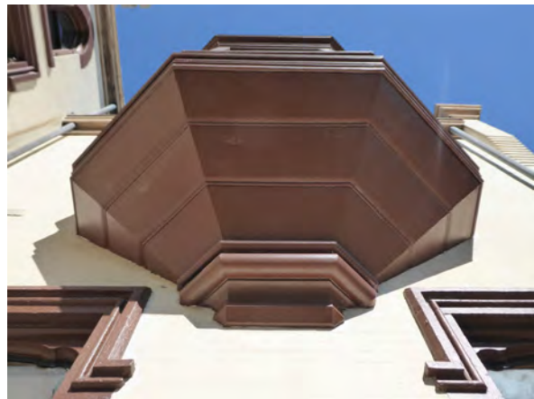
Photo 55: Base of oriel window.
