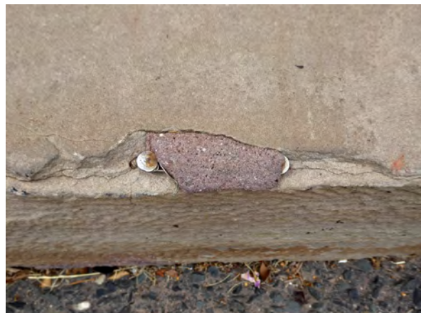
Photo 44: Cementitious patch anchored with nails at bottom step of entry porch.
