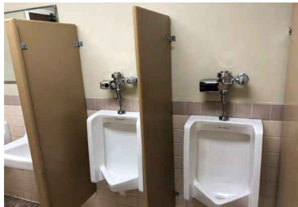
Photo 247: Urinals on east wall in Room 210.
