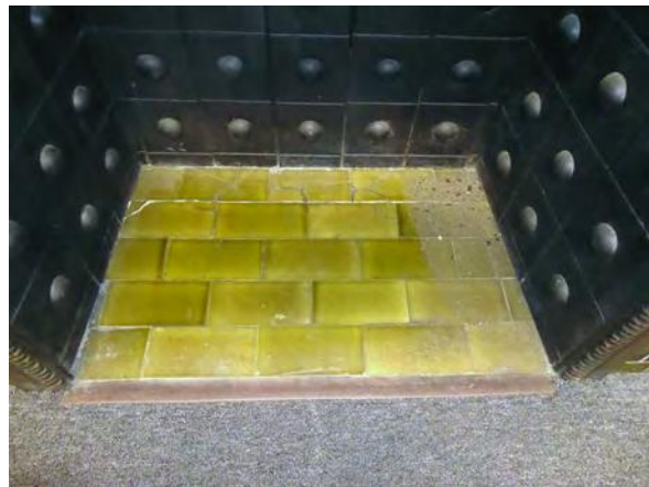
Photo 144: Ceramic tile floor with some cracking at fireplace.
