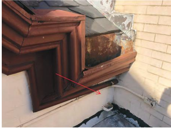
Photo 19: Missing Borough Hall downspout at Library Addition roof.
