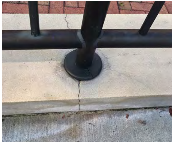
Photo 71: Crack on coping at railing post.
