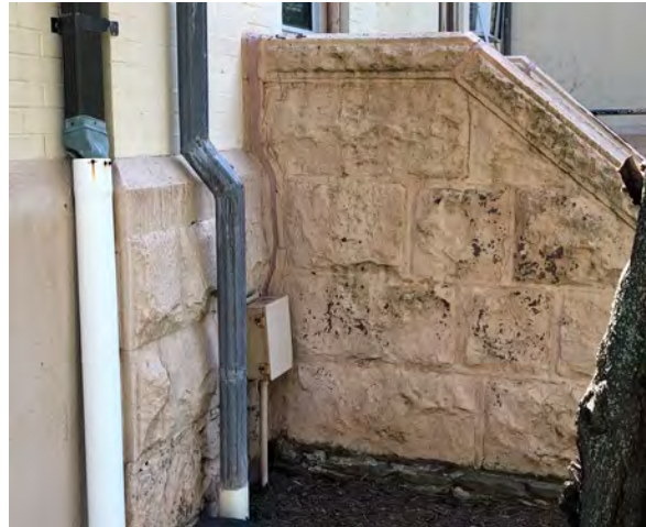
Photo 89: Separation of west entry stair side wall from building, filled in.
