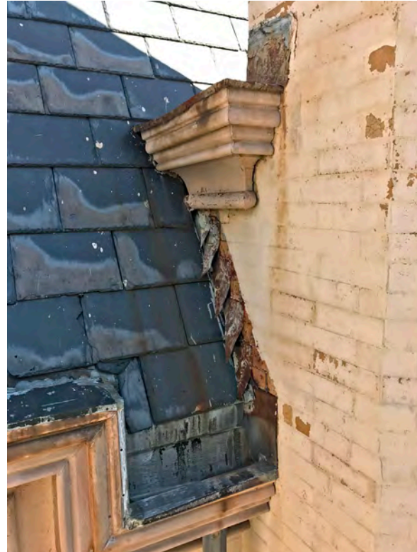
Photo 10: Example photo of deteriorated built-in gutter liner, wall flashing and cap flashing at Borough Hall. Taken from south elevation.
