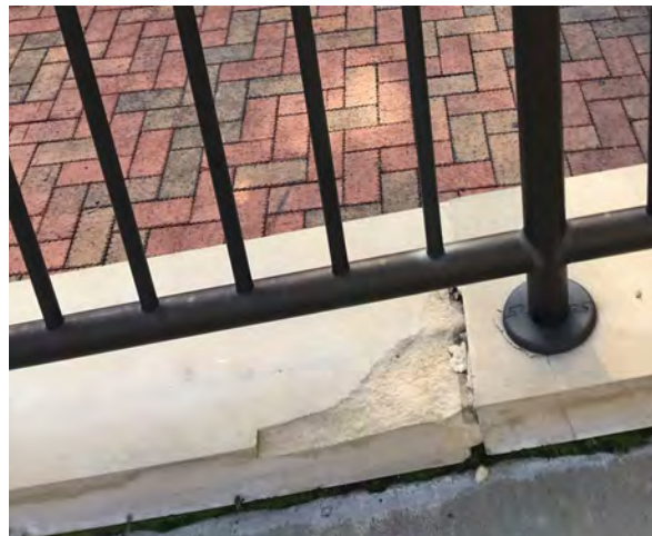
Photo 72: Spall on coping unit.
