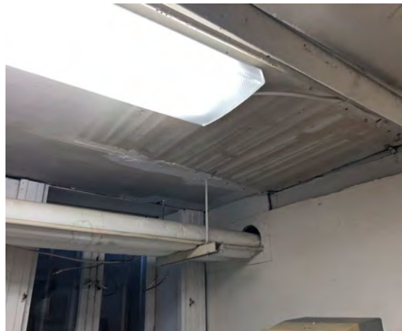
Photo 35: Water damage on the northeast corner of the ceiling.
