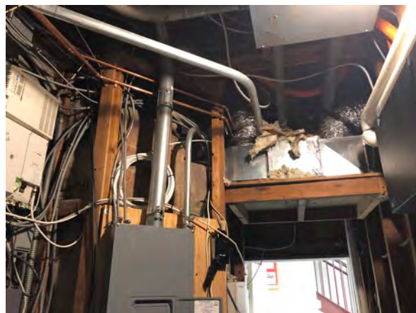
Photo 85: Wiring, piping, and duct at ceiling and walls in Room 020.
