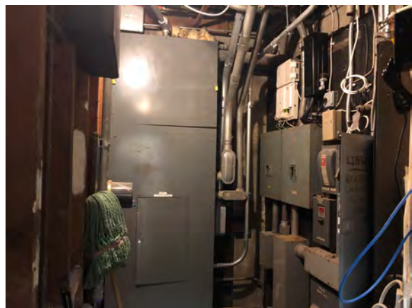
Photo 87: Electrical service equipment on north and east walls in Room 020.
