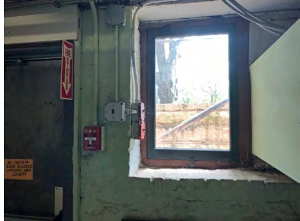
Photo 45: Window opening with awning sash and louvered duct on south wall in Room 011.
