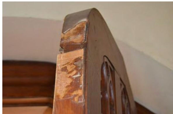
Photo 127: Abrasion and detached top wood veneer on door to stair tower in Room 103.
