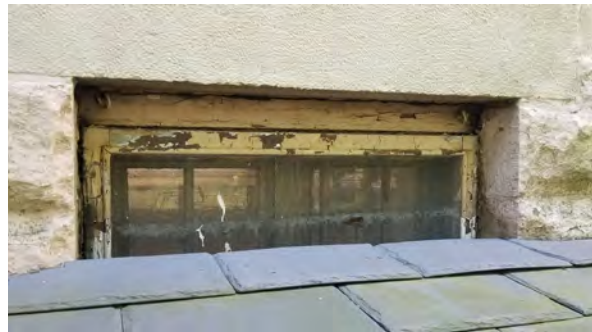
Photo 64: Typical condition of deteriorated foundation windows on north elevation of Borough Hall.
