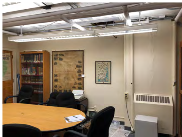
Photo 72: View north in Room 017. Note location of ceiling leak in center of photo.
