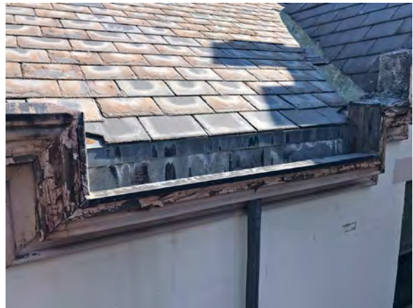
Photo 14: Typical condition of deteriorated wood cornices on Borough Hall.
