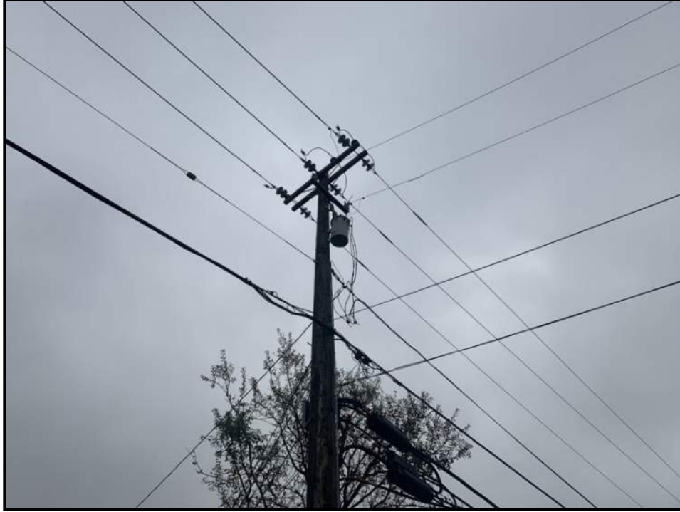
Photo 7: View of pole-mounted transformer located on the west portion of the Subject Property.
