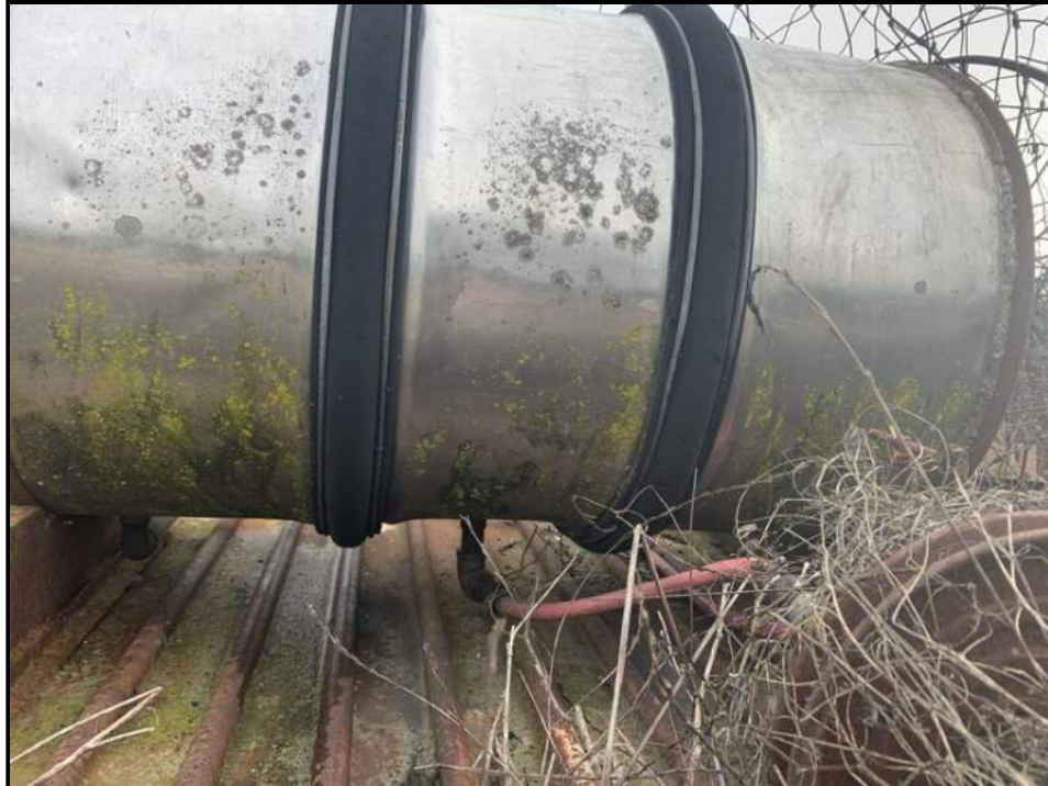
Photo 22: View of AST and associated piping located beneath the AST.
