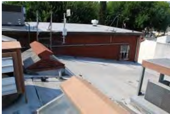
Figure 29: Roof, window at right side of north façade of second story, facing south.
