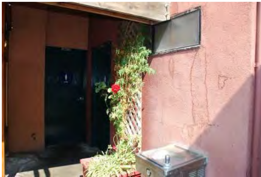
Figure 14: East facade, rear portion, south facade of first one-story mass where it meets the middle portion of the building, including restroom doors, facing northwest.
