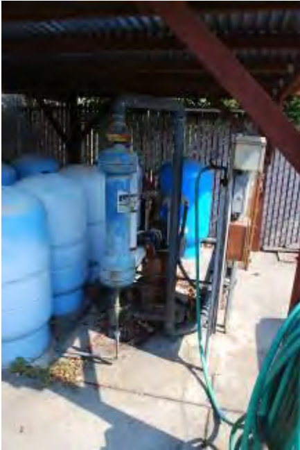
Figure 20: Utility yard at rear of building, containing well and pumps, facing northwest.
