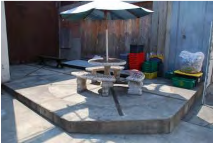
Figure 21: Utility yard at rear/west of building, concrete platform showing former footprint of cheese-making tanks, facing southeast.
