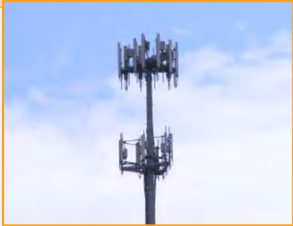
Typical Macro facility – industry standard sized collocateable facility with full compliment of radios
