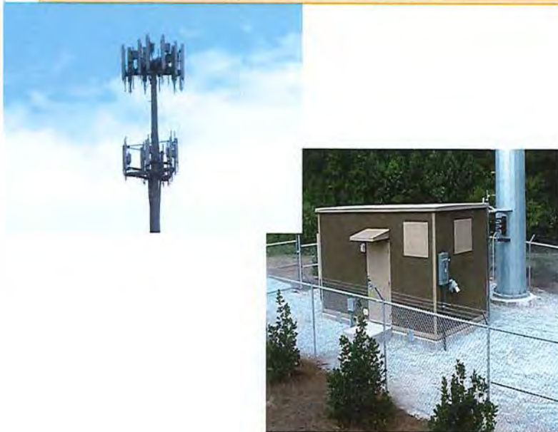
Typical Macro facility – industry standard sized collocateable facility with full compliment of radios
