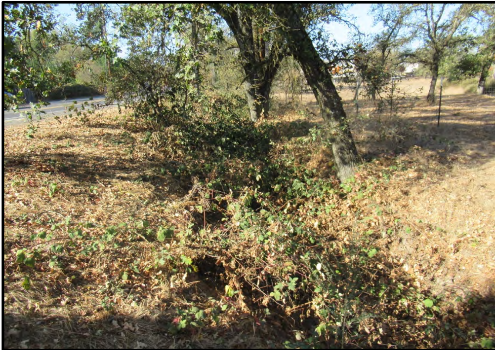
Roadside ditch just south of the south edge of the site, looking west down the ditch from the intersection of Napa Road and 5th Street; 11/22/19. This roadside ditch drains into the culvert under Napa Road.
